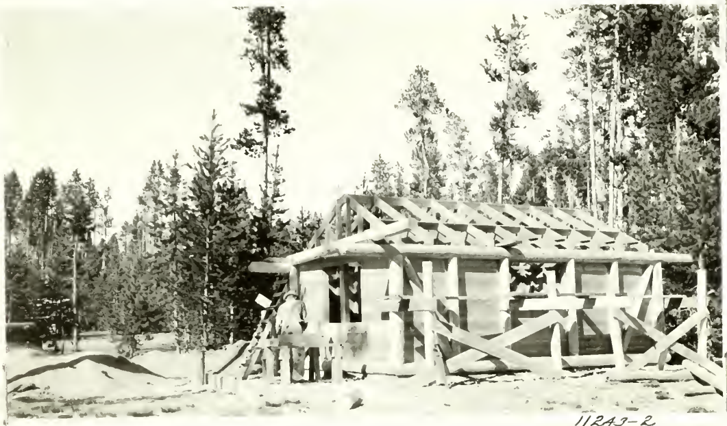
(1935) FP 146 Sewer System, Fishing Bridge. View of pump house being constructed under contract.
