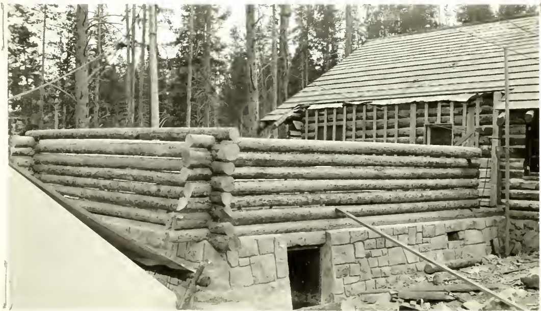
(1935) FP 138 Ranger Station, Addition, Canyon. View of annex being built under this project, to the existing Canyon Ranger Station.
