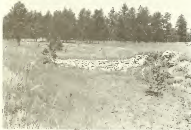
Figure 15.—A rock and wire check dam installed in 1936 was effective in 1983.
