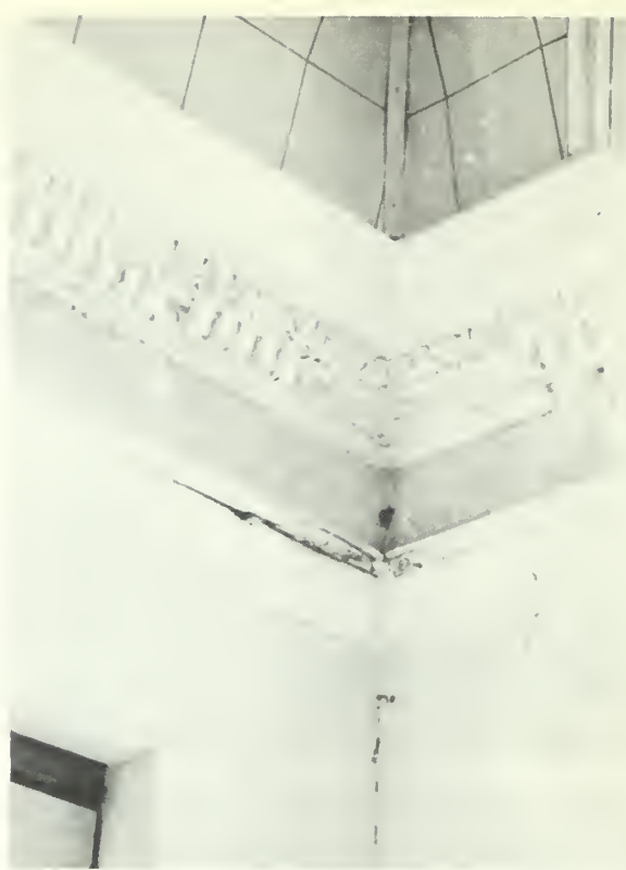
Fig. 11. The cornice of an Iowa courthouse has been severely damaged from a roof leak. In order to repair the ornamental plaster, a thixotropic rubber impression will be taken (with the paint build-up undisturbed). The efflorescence will be removed and fresh plaster casts installed so that egg and dart, dentil and leaf molding are perfectly aligned. Photo: National Park Service files.
