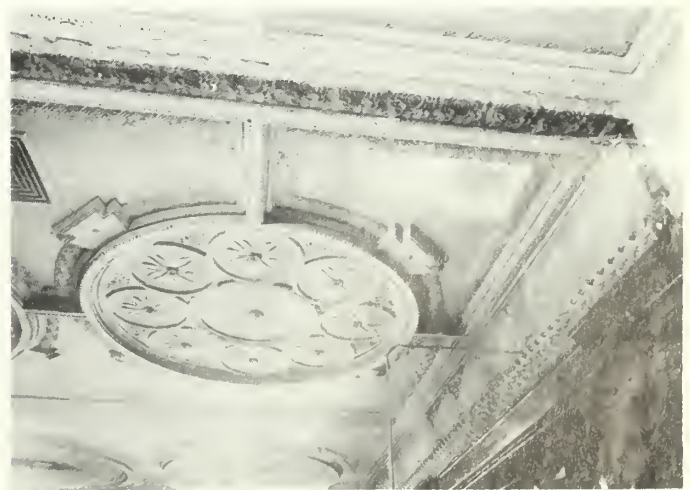
Fig. 16. The Auditorium Building, Chicago, Illinois, 1889, by Louis Sullivan. Earlier insensitive alterations were removed prior to restoration of the room. In the photo, a partition wall has already been removed; the electrical conduit and a ventilation grille followed. Plaster patching and painting were the final steps of restoration work. Photo: National Park Service files.
