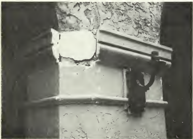
Fig. 14. A mitered portion of this impost capital abacus has fallen, revealing the plaster adhesive material. Repairs are made by obtaining a section through the abacus, making a bench-run length, cutting, fitting, and readhering the missing piece. Finally, the joints are pointed. Photo: Lee H. Nelson, FAIA.
