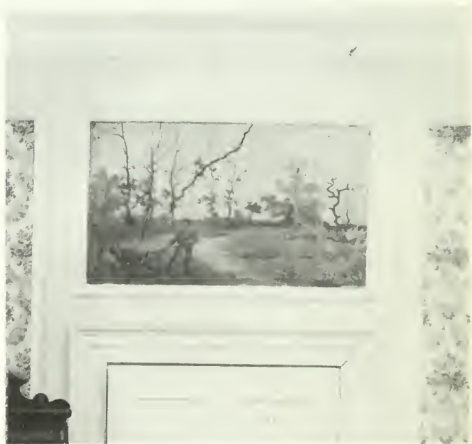
Fig. 12. Settlement caused stress cracking through both flat wall and ornamental plaster. Repairs to the cornice involve chamfering the stress cracks to a "V groove" and patching with a mixture of gypsum and lime. The cornice can be countersunk-screwed to its substrate to prevent further movement. Screw heads are then plastered over. The crack running through the painting will need to be filled carefully, and the painting restored by a trained conservator. Photo: Jack E. Boucher, Historic American Buildings Survey.
