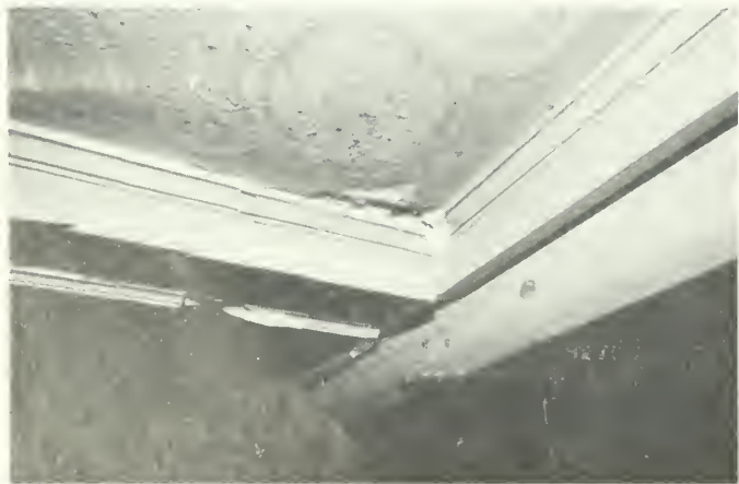
Fig. 10. Structural settling has caused this ceiling to deflect. Prior to restoring the damaged plaster and final repainting, a structural engineer experienced in historic preservation will be engaged to shore-up the ceiling from below and reattach the sagging ceiling plaster with the joists above (see also Fig. 17 under Immediate Action.) Photo: National Park Service files.
