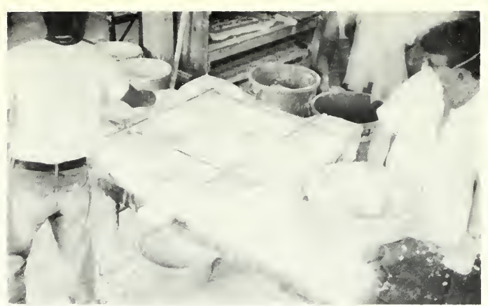
Fig. 8. Casting a Coffering Unit. Ceiling coffers are made the same way today except, historically, a hide glue mold was poured over an ornamental model whereas today urethane molding rubber is used. Now, as then, the plaster casts are made with steel channel irons embedded on the back of each panel. The coffers are hung from carrying irons fixed to the ceiling above by means of twisting wires to level each coffer to its neighbor. Afterward, the panels are fastened together and the joints pointed with plaster. Photo: David Flaharty.
