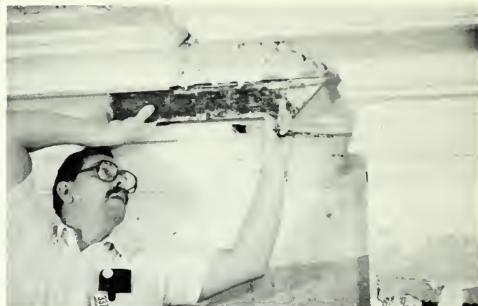
Fig. 5. Mitering a Plain-Run Cornice. Mitering requires great dexterity using the miter rod. In this case, a return at a chimney breast is tooled using an infill of gypsum and lime. Internal and external miters are required with the internal being the most difficult. Another method is to run a length of cornice (using the same blade) on a bench and set it in place, later to point the joints. Photo: Old-House Journal.
