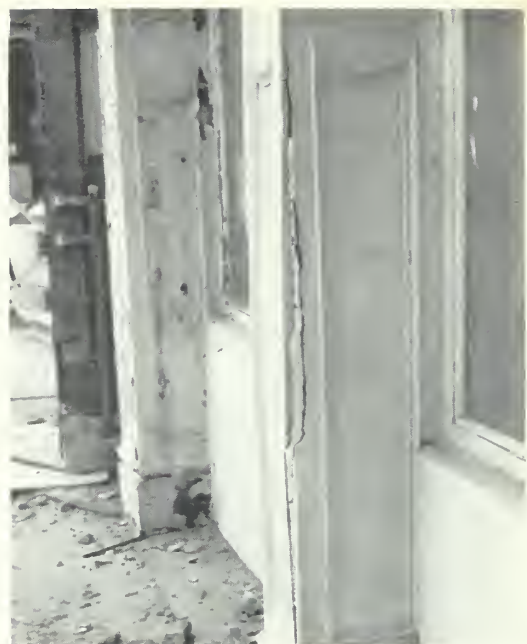
Fig. 11. Major cracks in the piers of this cast-iron storefront in Galveston, Texas resulted from the transfer of load onto the iron from internal brick piers eroded by rising damp. This crack was inappropriately filled with concrete, which trapped moisture and accelerated internal corrosion, pushing the iron further apart. Photo: Ford, Powell & Carson.
