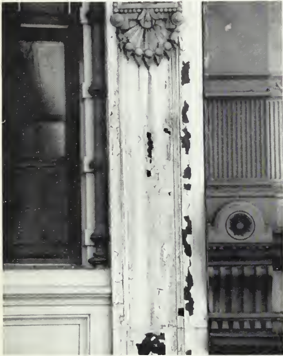
Fig. 14. Major problems can result if work is undertaken without proper sequencing and precautions. On this building, a strong alkaline paint remover was used, and apparently was not adequately rinsed or neutralized. Over a period of months, the newly applied paint began to peel and streaks of rust appeared on the iron. Photo: Kim Lovejoy.
