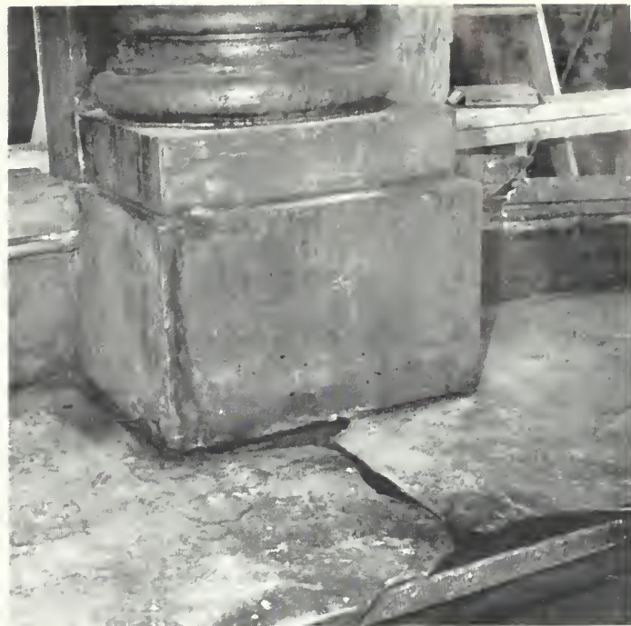
Fig. 12. Paint stripping exposed a large defect under a faulty patch at a joint of this wide cast-iron water table. The damage can be repaired mechanically by splicing in a cast-iron replacement piece. Photo: Peter Jensen, Kapell and Kostow Architects.
