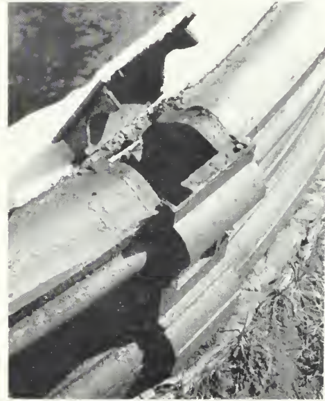
Fig. 9. Galvanic corrosion occurred where a patch of copper was installed alongside the cast-iron cap at the base of a fountain. The use of terne-coated stainless flashings with appropriate caulking would have been a more suitable repair. Photo: John G. Waite.
