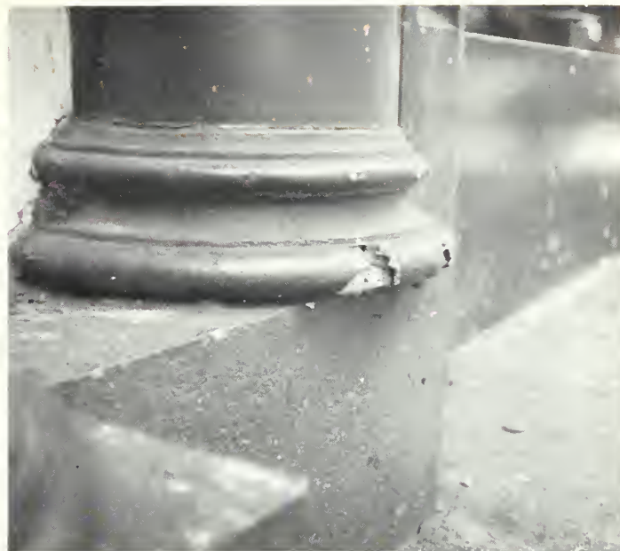
Fig. 20. The location of the feature must be taken into account if a substitute replacement material is being considered. This lightweight fiberglass column at street level sustained damage from impact within a few years of installation. The great strength of cast iron makes it ideal for storefronts and elements that must withstand heavy use. Photo: Building Conservation Associates.
