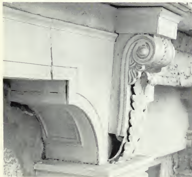
Fig. 8. Structural cracks, gaps at joints between components, and a large opening where part of the console bracket is missing are the problems evident in this cast-iron assembly. Photo: Ford, Powell & Carson.
