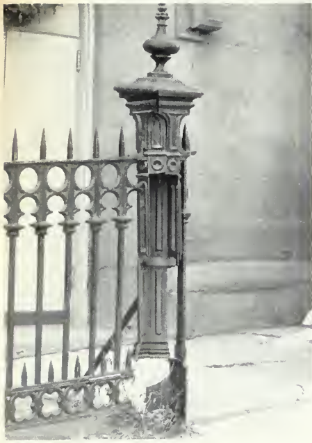
Fig. 7. Despite an impact that shattered the main castings, this fence post remains upright, demonstrating the great strength of cast iron. Originally, the post was held together by a long bolt that extended from the finial to the base. Photo: John G. Waite.
