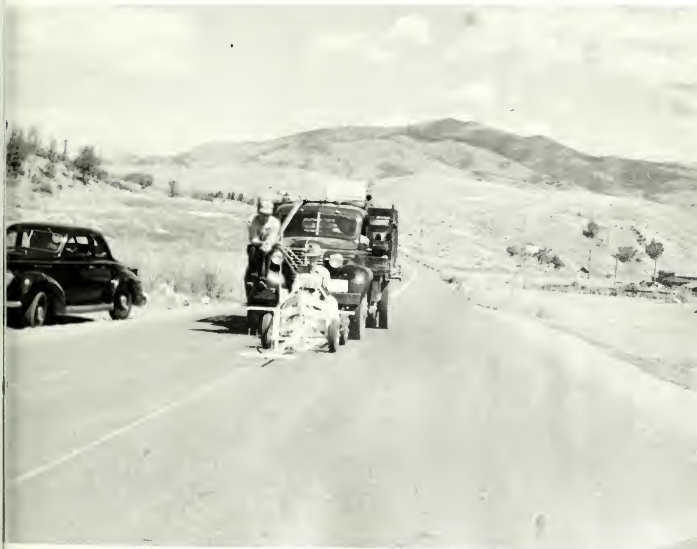
Road striping machine in operation near Mammoth Hot Springs Yellowstone National Park July 28, 1941
