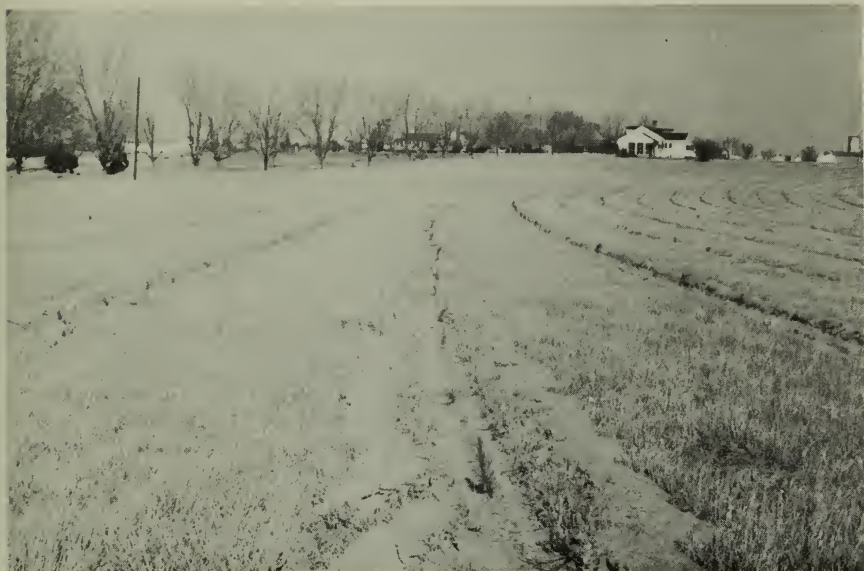
Fig. 2. Site preparation on heavy sodded area, showing furrows and newly planted seedlings.
