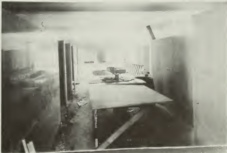
Figure 12: The Interior of the Hale during Remodeling (Men's Bath Hall), 1914 (Source: National Archives, Natural Resources Division, R.G. 79)
