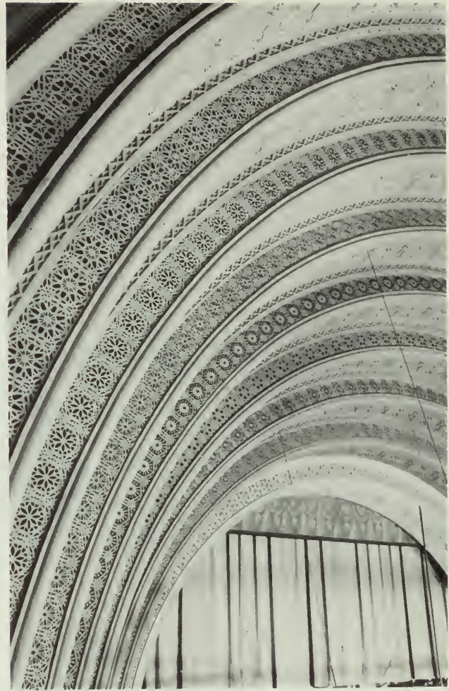
Detail from: SCHILLER BUILDING (later Garrick Theater), 1891-92 (demolished 1961). ADLER AND SULLIVAN, architects. Photograph by Richard Nickel and Aaron Siskind for AIA Chicago Chapter.
