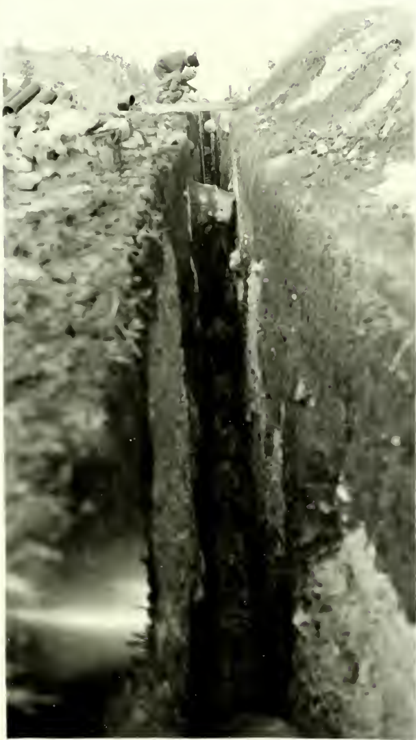
Sewer System - CCC Job No. 7. Fifty per cent of 8" sewer main for Mammoth Camp Ground completed.
