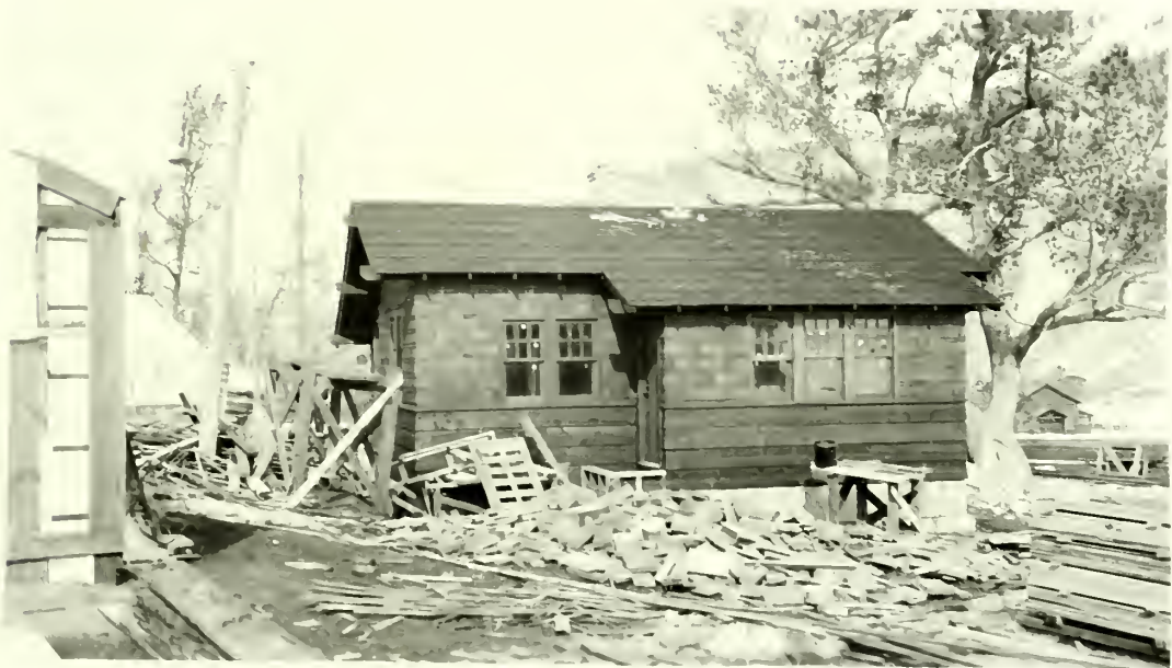
Employees Cottage - CCC Job No. 412 - Mammoth. Two cottages of this type are 90% complete.
