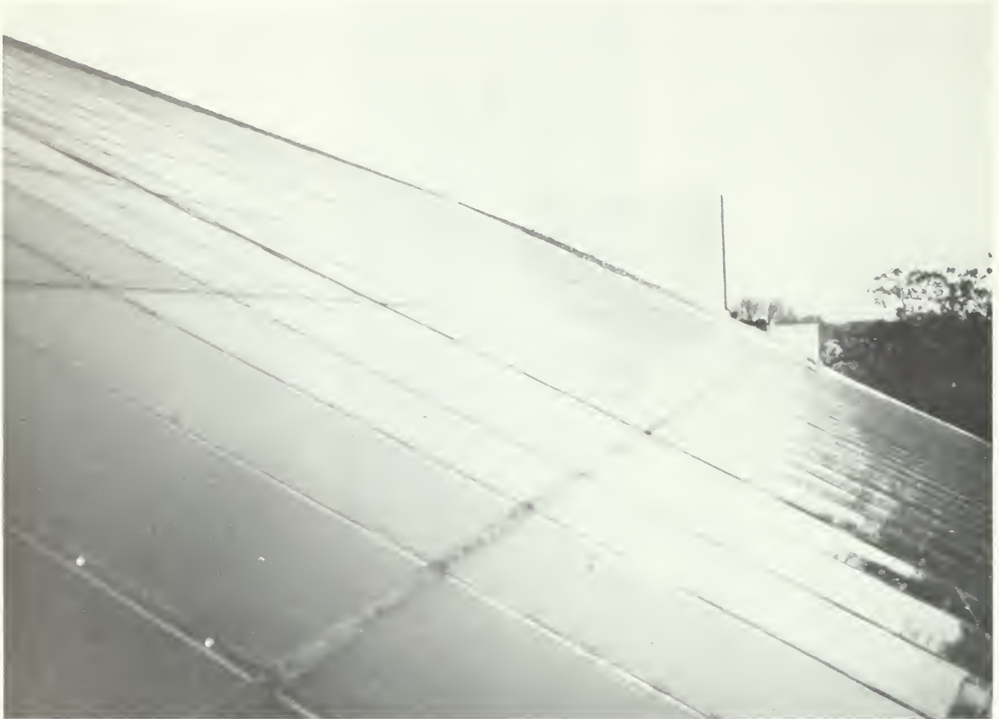
A federal grant enabled the state to place an active solar system on the 10,000 square-foot sloping roof of Deer Creek State Park Lodge.
