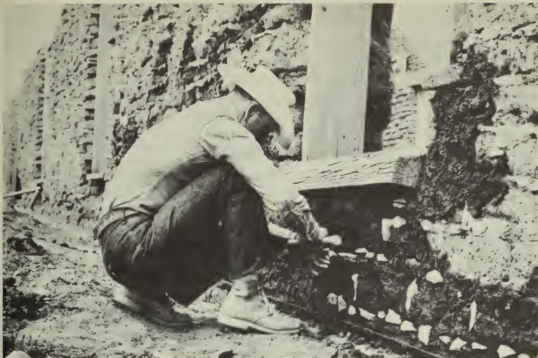
The adobe barracks were among the first buildings to require attention when the National Park Service's rehabilitation program began in 1963. Here a workman shores a weak wall.
