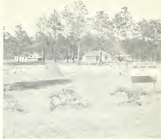
The construction of a training center and sewage disposal plant is underway at the Waycross State Forest.
