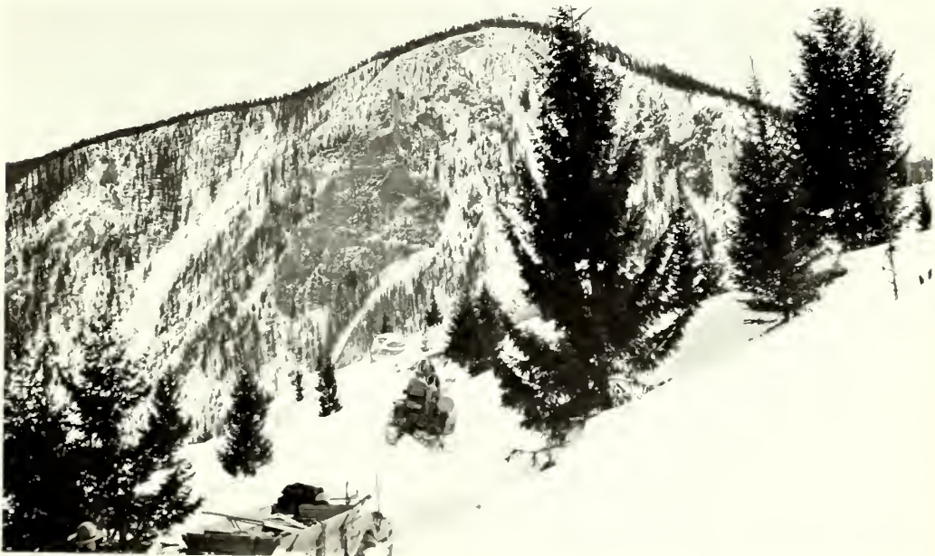
Taken April 7, 1932. Opening road near the Hoodoos. Bansen Peak in background. A caterpillar 60 was used on this work and it was necessary to blow out many large drifts.
