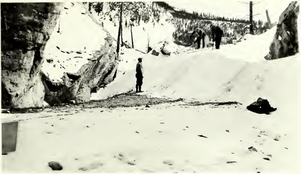
Taken April 7, 1932. Opening road near Silver Gate. Digging holes for placing powder to blow large drift south of Silver Gate.
