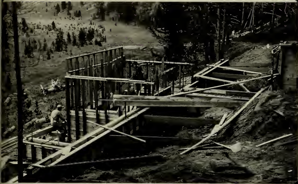
Project 423 - New Incinerator at Fishing Bridge. During construction about the middle of September. Putting up forms.
