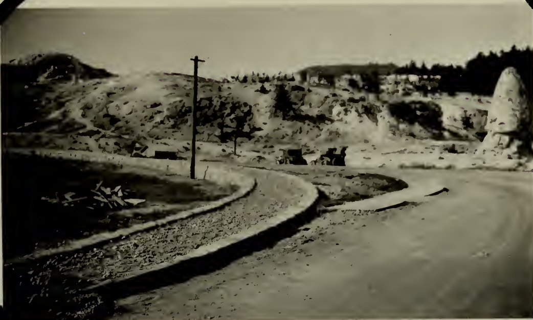
Project 502.26 - Sidewalk at Mammoth. Between Lodge & Hotel. Showing stone curb and unrolled subgrade. Note old sidewalk and improved intersection.
