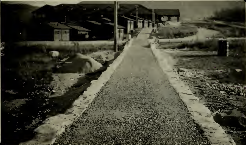
Project 502.26 Sidewalk at Mammoth. Base course sprayed with asphalt. Pictures of finished sidewalk will be shown in later report.
