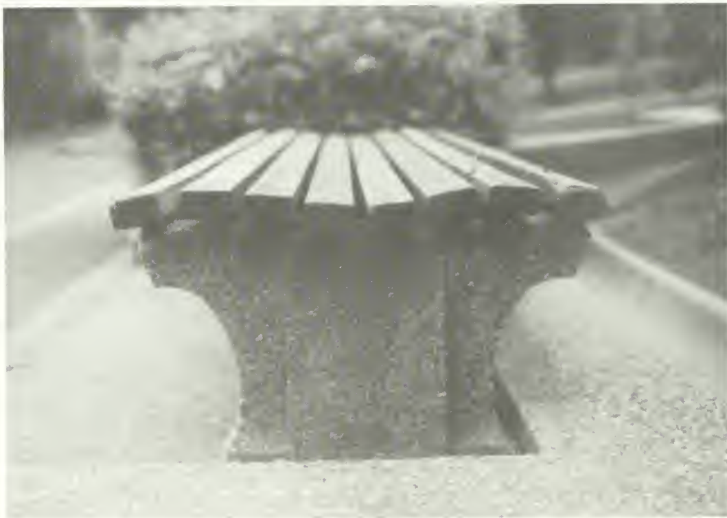
The original bench slat attachment detail on these contoured benches is both elegant and difficult to maintain. It is critical to develop a practical method of attachment that is consistent with the historic character of the benches.
