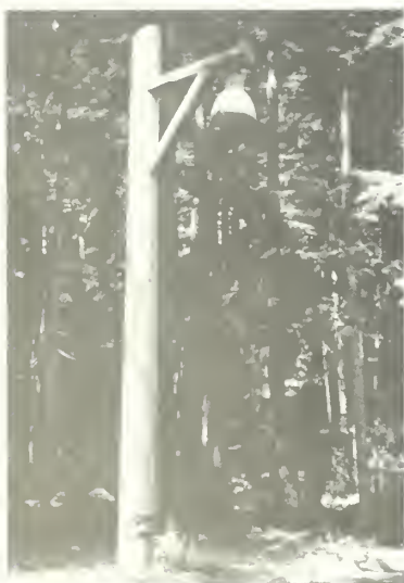
Street Lighting at Newhalem Campground, North Cascades National Park
