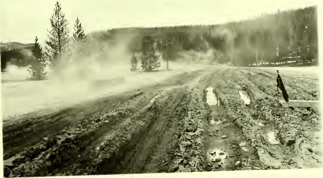
Subgrade failure on newly constructed Firshole Cascades-Old Faithful section. Photo just back of auto in background of preceding picture.
