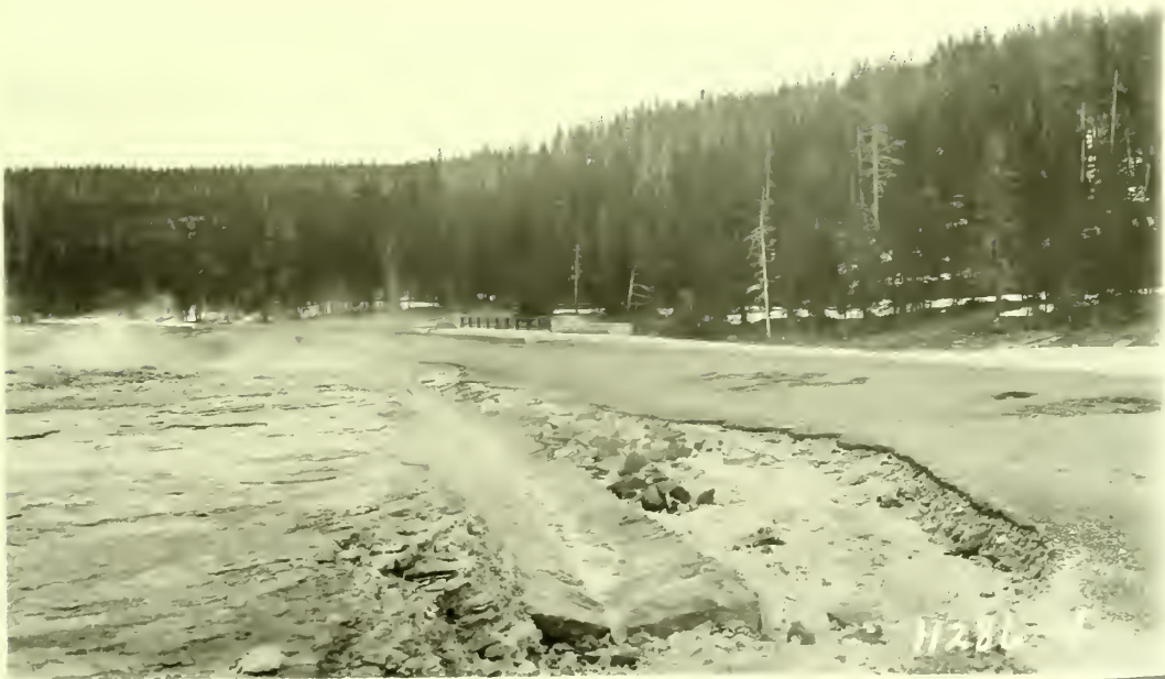
Washout of paved gutter and oil surface in same vicinity as preceding picture.
