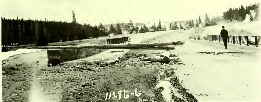
Washout of bridge approach at Firehole River near Riverside Geyser.
