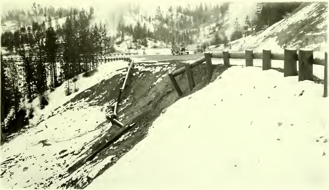
Washout of new grade on Canyon-Lake section of Mud Volcano.
