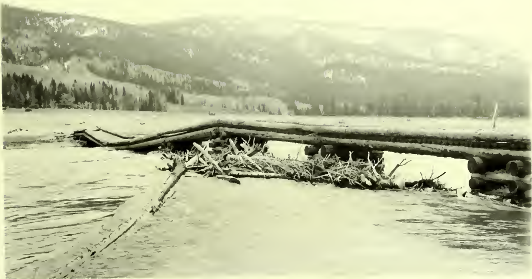
Trestle Bridge across Snake River, near South Entrance, damaged by flood waters and drifting debris.
