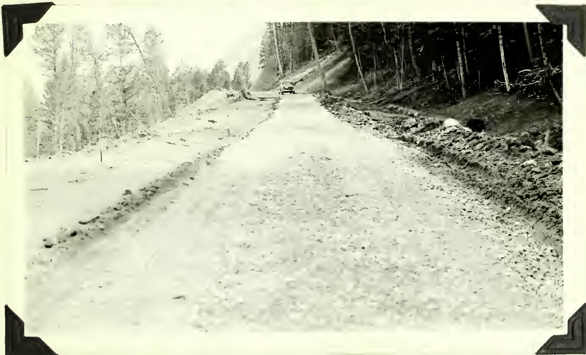
Slippage of fill on Mammoth - Tower Junction section.
