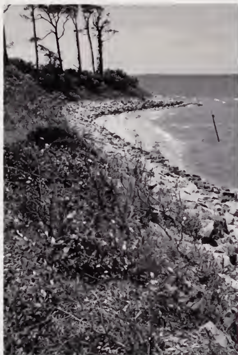
FIGURE 17. Stone rip rap is also used along some areas of the shoreline to control erosion. Source: JMA, Inc., 2009.
