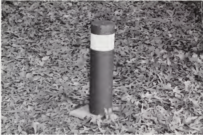
FIGURE 77. Small metal bollard light located throughout the visitor center area of the park. Source: JMA, Inc., 2009.
