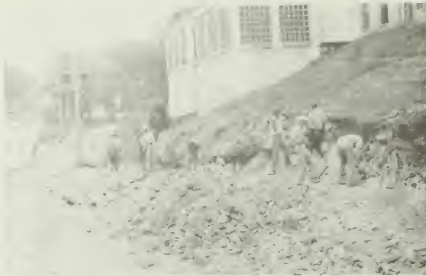
Figure 5. Grand Promenade Cut near Army and Navy Hospital, early 1930's (Source: Hot Springs National Park)
