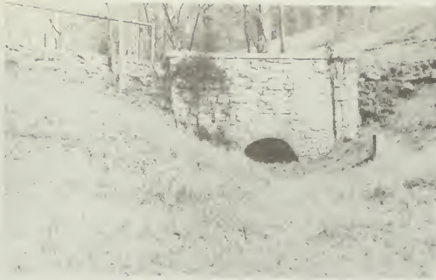
Figure 23. Stone Culvert on Hot Springs Mountain, date unknown (Source: Hot Springs National Park)
