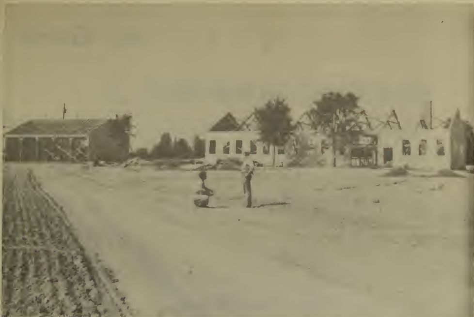
SIGNS OF PROGRESS-- Construction of packing and equipment sheds at the new nursery are nearing completion. Seedlings will be graded, counted and packed for shipment in the building on the right.
