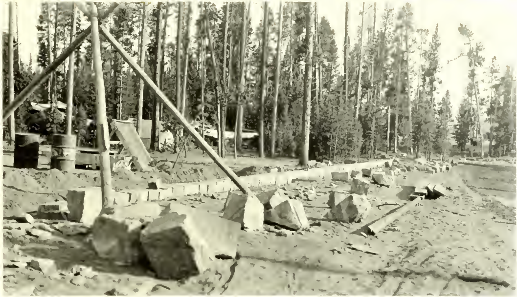
F.P. 224.8 - Campgrounds Roads, Fishing Bridge Section of parking area curb.
