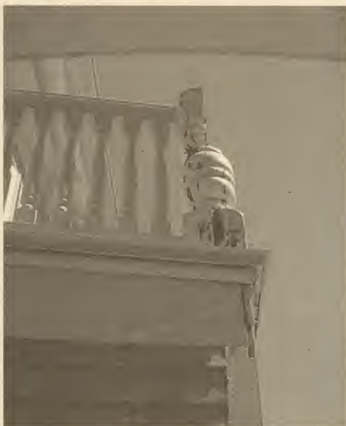
Termite damage at Perseverance Hall, New Orleans
