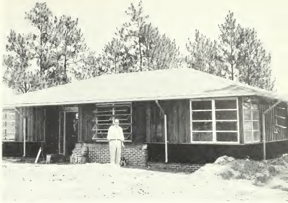
NEW EIGHTH DISTRICT HEADQUARTERS-- G. W. Lavinder, Eighth District Forester, Georgia Forestry Commission, inspects the new district office being built at the headquarters site south of Waycross on U. S. Highway 1. Offices for district headquarters personnel, a radio repair room, and a storeroom are included.
