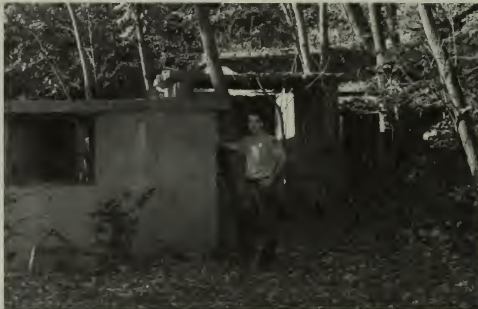
Deteriorating structure hides a large, 6' x 10' open portal. Photo by Robert Sullivan.
