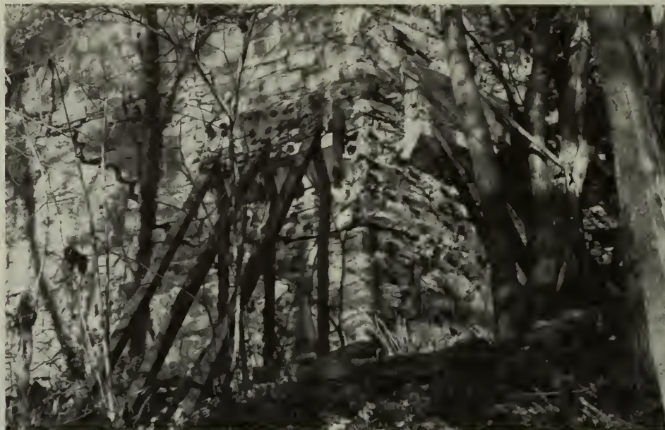
Deteriorating stone wall from the Ames Mine site. Photo by Robert Sullivan.
