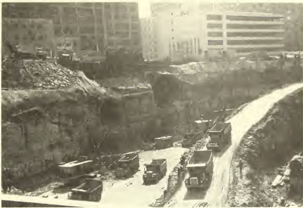
PHOTO 20: EXCAVATION FOR THE FOUNDATION OF THE U.S. STEEL BUILDING, PITTSBURGH, 1966. The excavation uncovered the tunnels of the Pennsylvania Main Line Canal and the Pennsylvania Railroad. This extraordinary juxtaposition illustrates the way in which transportation helped lay the city's foundation and also symbolizes the historic link between the transportation and steel industries. Courtesy of the Historical Society of Western Pennsylvania.
