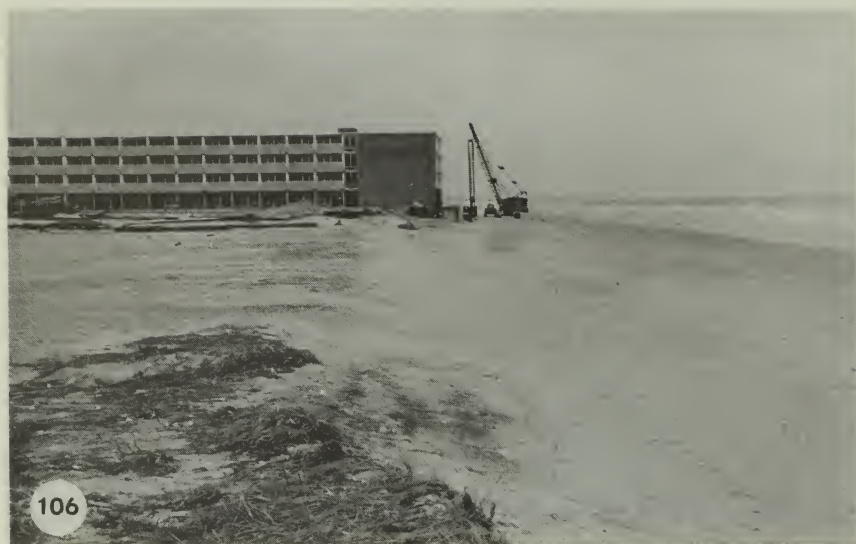
Fig. 106. A resort motel under construction at Wrightsville Beach, North Carolina. The high tide line is in the foreground.
