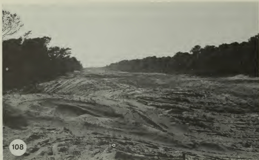
Fig. 108. Road cut through an outstanding maritime forest on western Bogue Banks.
