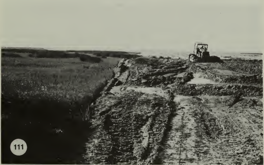
Fig. 111. Marsh adjacent to the same bay is being filled to make a parking lot for the boat launchers. This sort of thing would presumably not be done today.
