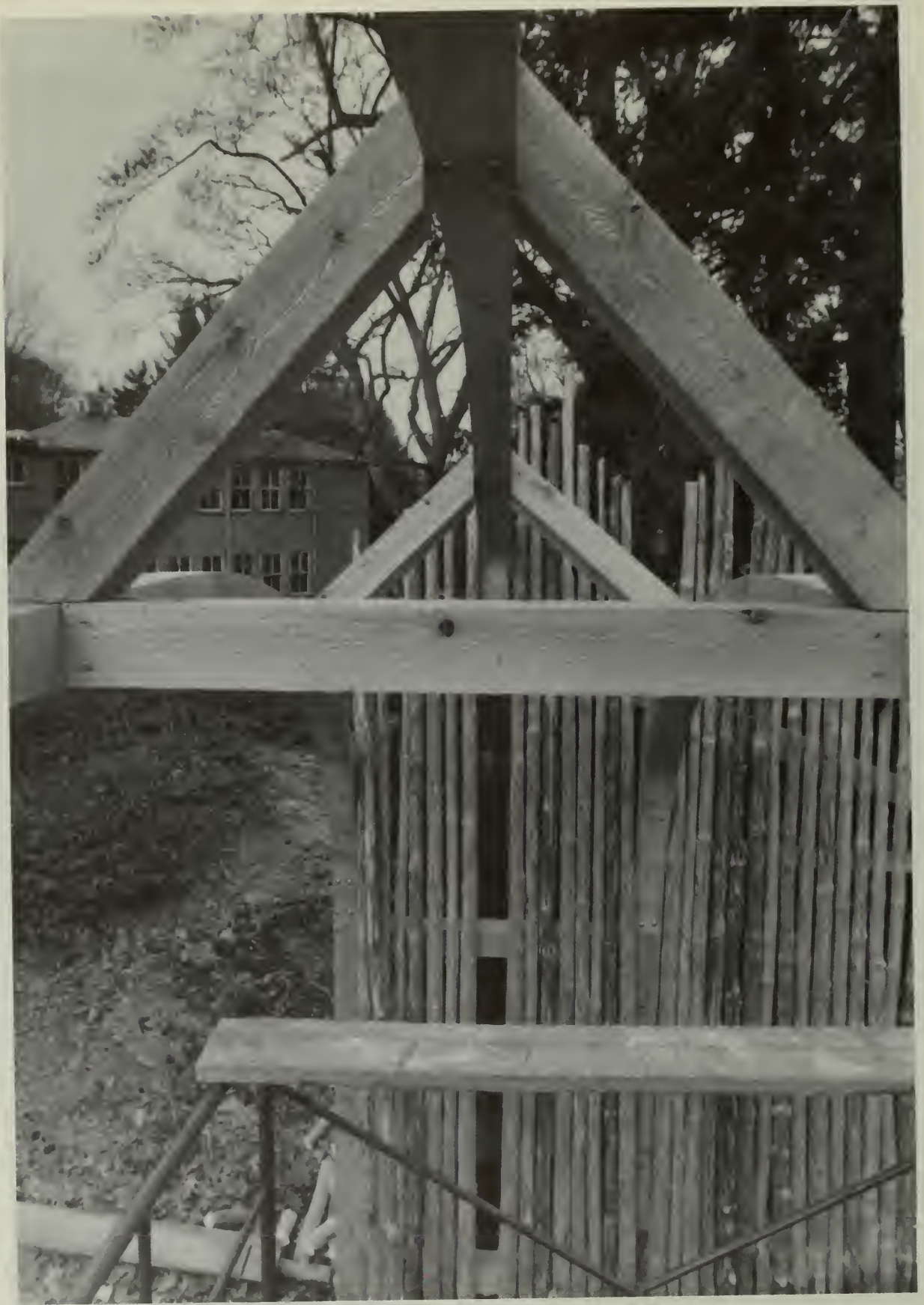
Figure 54. Spruce pole fence: reconstruction of the front driveway arch during the 1984 rebuilding.
