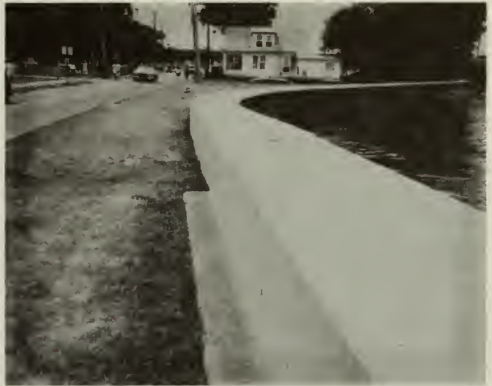
Fig. 32 View of the north seawall constructed over the earlier 1934-35 seawall [by author].
