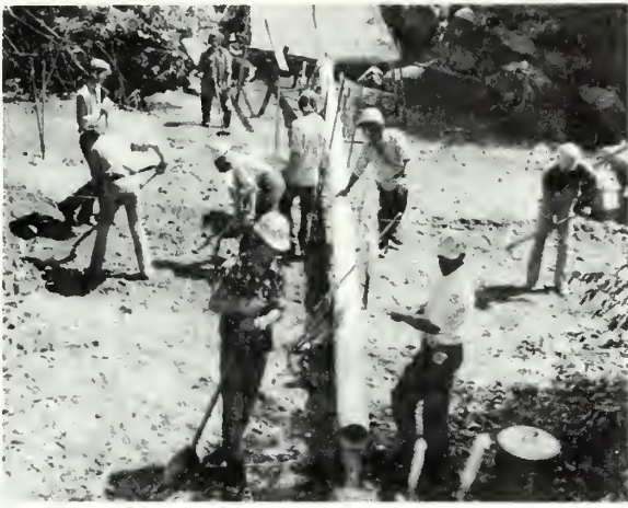
Youth Conservation Corps enrollees excavating fish trap construction site for California Cooperative Fishery Research Unit. Photo by Roger A. Barnhart.
