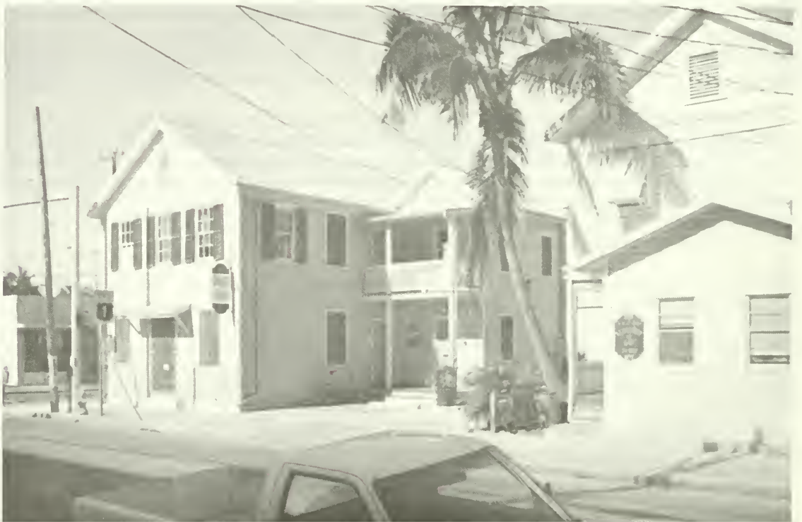
2. With the removal of the staircase there is no longer an indication of the second floor's independence from the first. The two floors of the ell addition appear to be functionally integrated.
