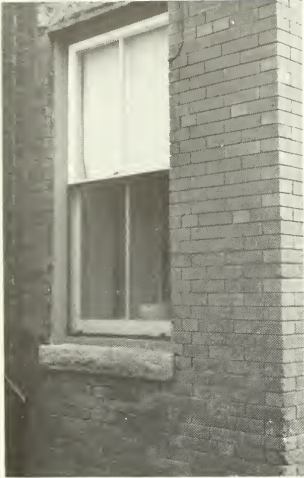
5. New wood replacement window as approved. If possible further refinement (although not required in this case) would have been to install the half screen on the inside rather than on the front of the upper and lower sash.
