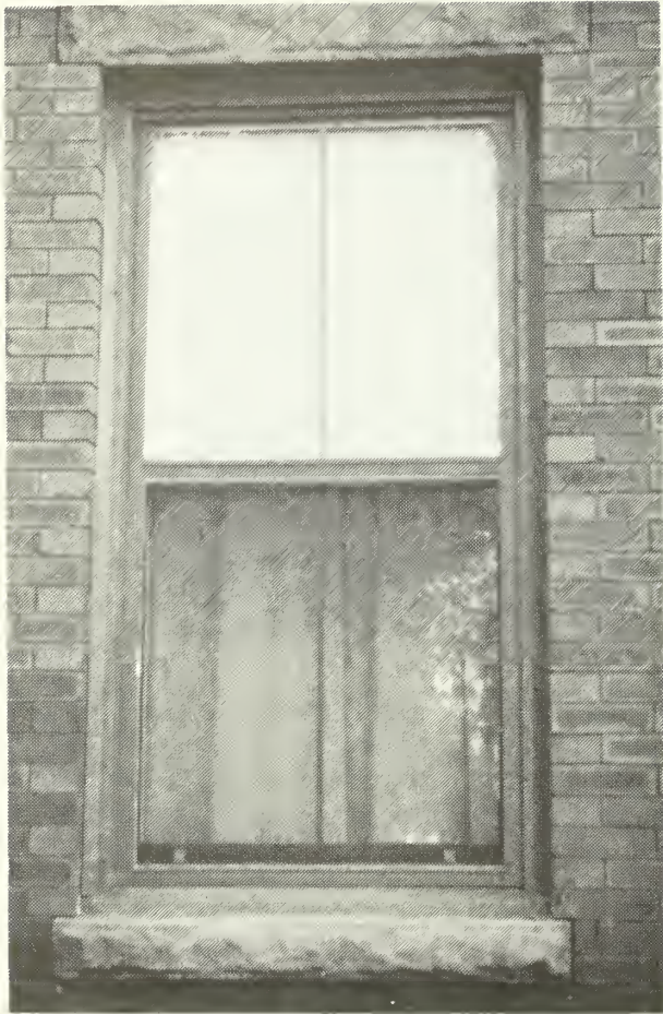
3. Post-rehabilitation photograph of aluminum replacement window. The vertical muntin was sandwiched within the insulating glass and the double-hung appearance changed since the screen panel was installed directly below the fixed upper sash.
