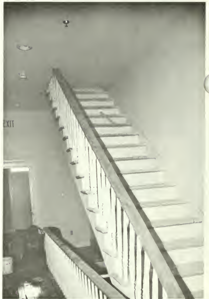
11. Post-rehabilitation view of original staircase maintained as a part of rehabilitation, but fourth floor is floored above, preventing access.
