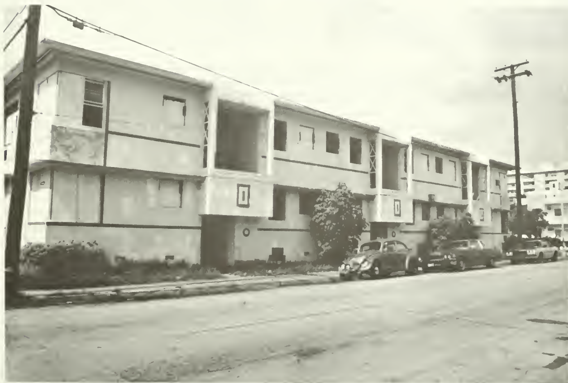
2. The street elevation of the building where patch repair work has already begun shows the decorative panels of local stone under the second story windows at either end of the building.
