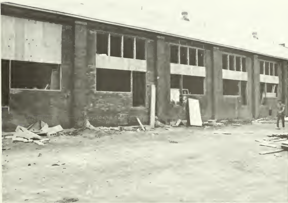
5-6. The rear elevation of the drill shed during rehabilitation. Note the extensive loss of brick, and how the character has changed with the removal of the multi-paned wood sash and the creation of large openings.
