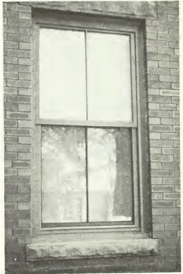
4. Aluminum replacement window with a wood mock-up of an applied unglazed sash frame and muntin placed over the upper aluminum sash. The applied frame and muntin look like temporary add-ons, rather than matching the historic sash.
