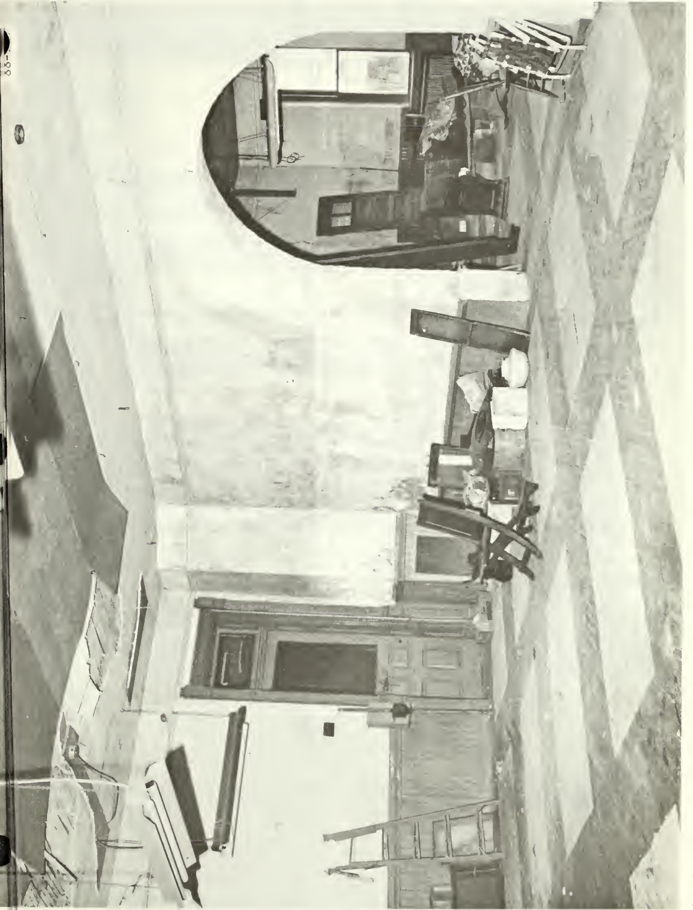
3. View of interior first floor classroom prior to rehabilitation. Arched opening between classrooms was added after original construction.
