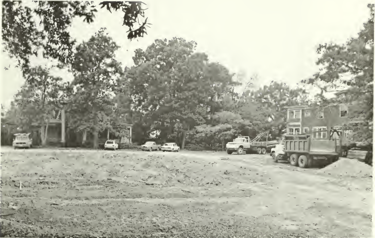
3. The front yard of the mansion has been prepared for the relocation of the neighboring house, seen at right.
