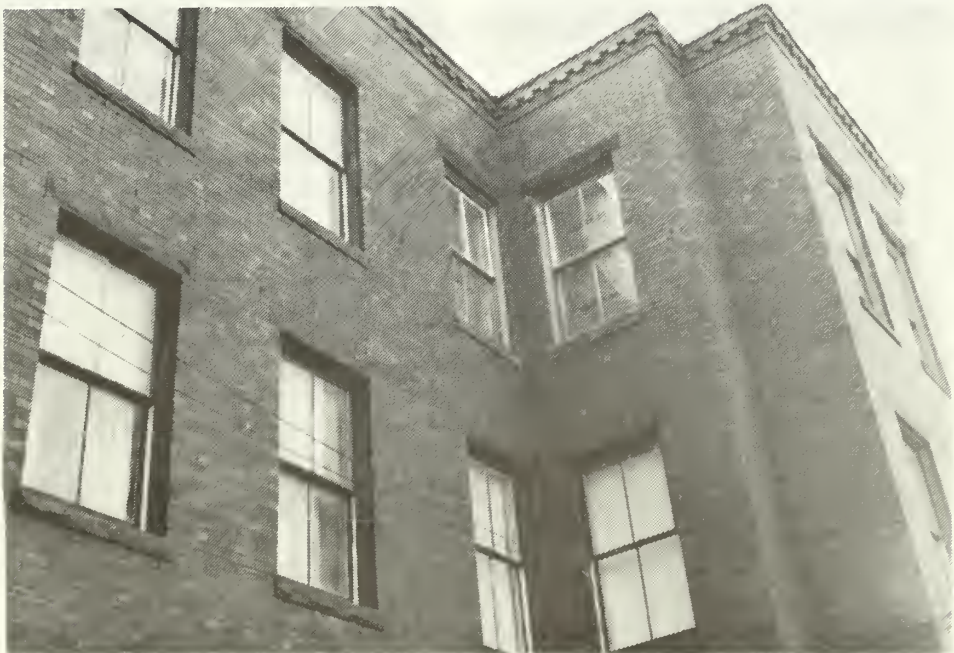
2. Pre-rehabilitation photograph of historic two-over-two double-hung windows that had a thin vertical muntin and wooden molding (brick molding) around the frame.
