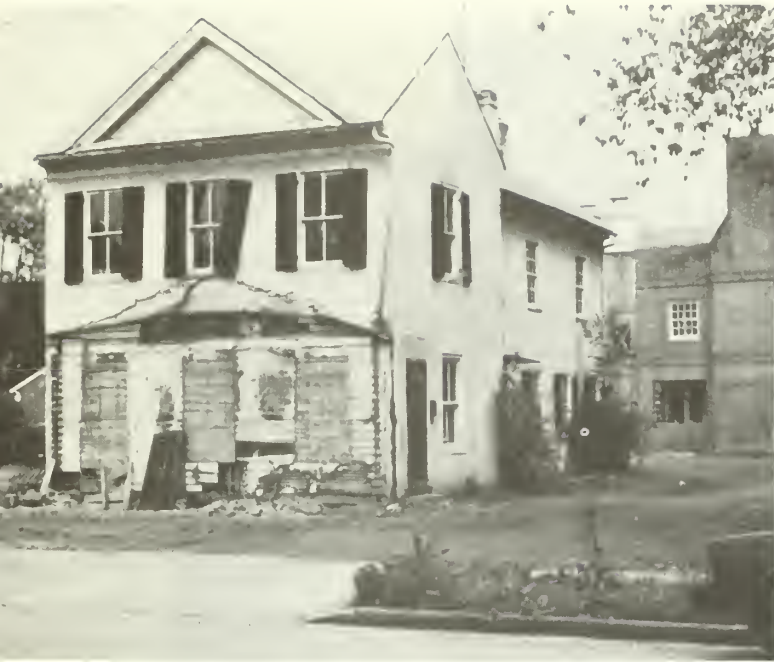
1. Front and side elevations of a ca. 1865-1870 wood frame building prior to rehabilitation. Stucco had been applied over the exterior wood at a later date and had caused rotting and termite infestation of historic wood. The building was certified as meeting Part 1 integrity requirements in its deteriorated and damaged condition.
