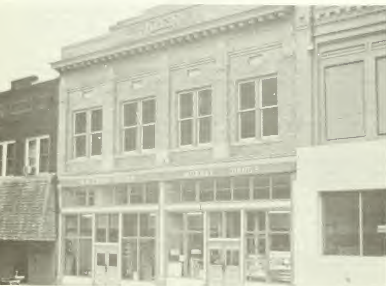
4. View of storefront after rehabilitation showing conjectural appearance of the original storefront — note inappropriate detailing of the transoms and small size of the doors.
