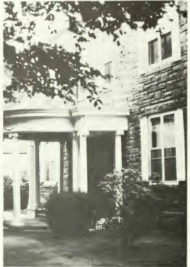
5. A photograph of a portion of the primary facade reveals a highly decorative porch, but also shows the nonhistoric concrete veneer, and aluminum sash and shutters.
