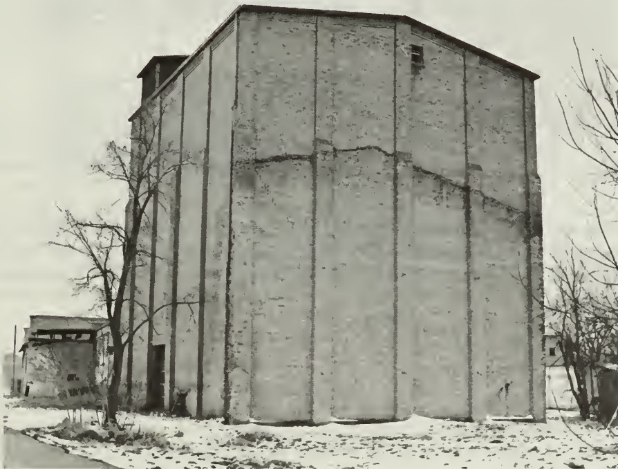
2. Ice storage house prior to rehabilitation. The massive brick structure was historically designed and constructed to be windowless on all four sides in order to enhance thermal efficiency. (The one opening seen near the top of the building is a small attic vent).
