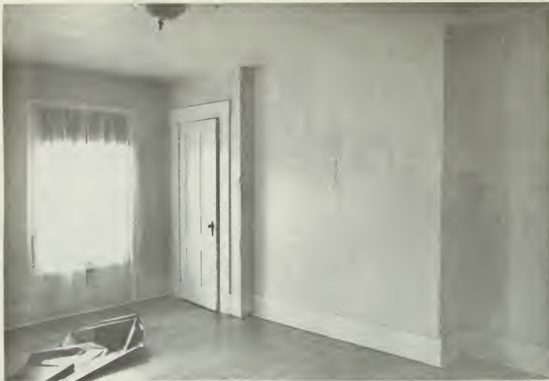
3. A typical room prior to rehabilitation. The room is defined by its flat ceiling, rectangular space, and simplicity of detailing.
