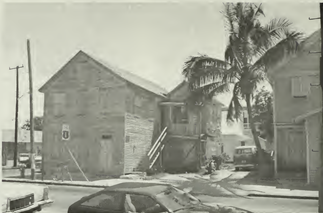
1. This view shows the exterior staircase in place before rehabilitation. Although this staircase was a replacement of the original, the feature was significant because it had remained in the same location and because it announced a separate use and function for the second floor of the ell.
