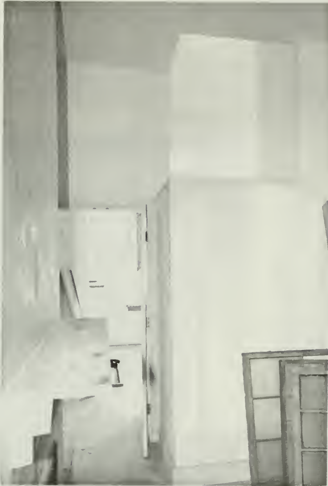
10. Work in progress on third floor showing penetration of wall between historic bedrooms, new staircase inserted in room and view to fourth floor above.
