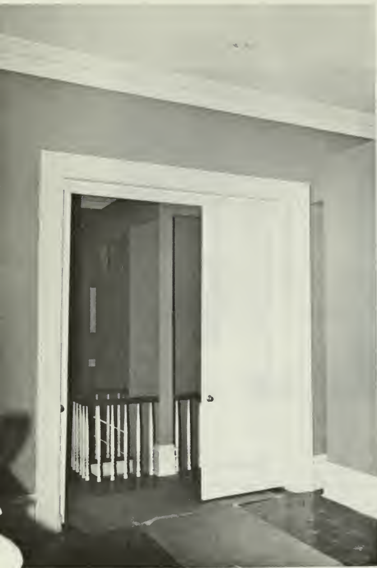
5. Post-rehabilitation: 2nd floor. Note new staircase and partition in center parlor room, new freestanding partition to the right of parlor door in front room.
