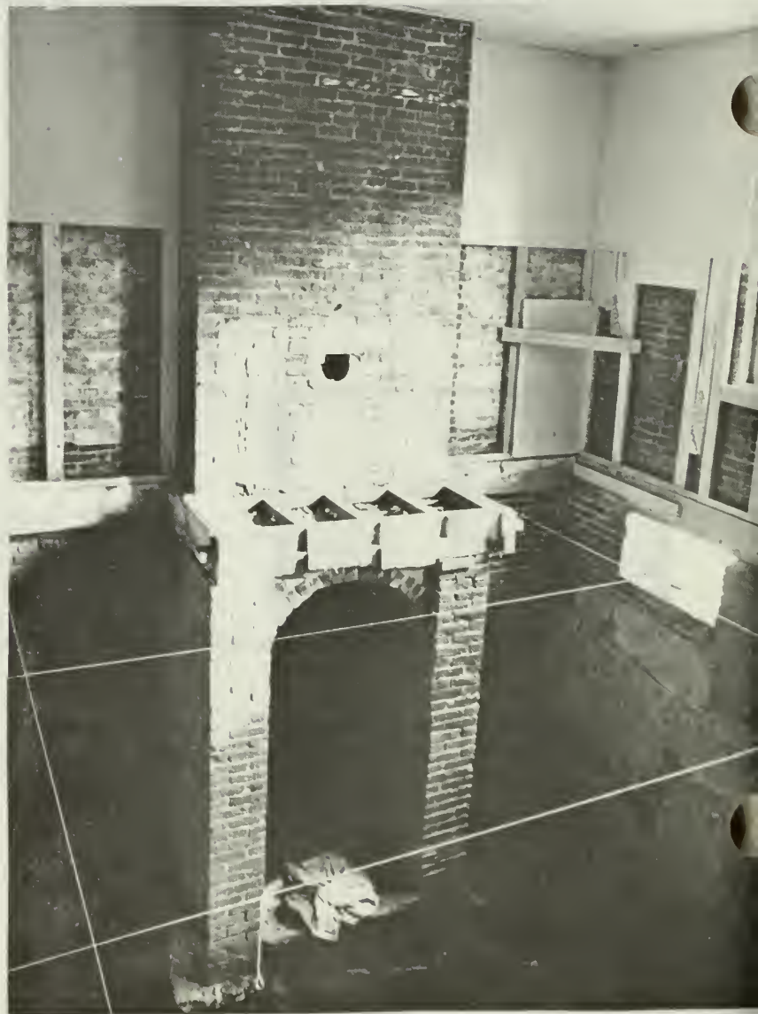
4. As part of the rehabilitation, the historic space was dramatically redefined by removing the first story floor, revealing the basement level. Two separate rectangular spaces were then made into one rehabilitated living unit. This inappropriate treatment violated both Standards 2 and 9.
