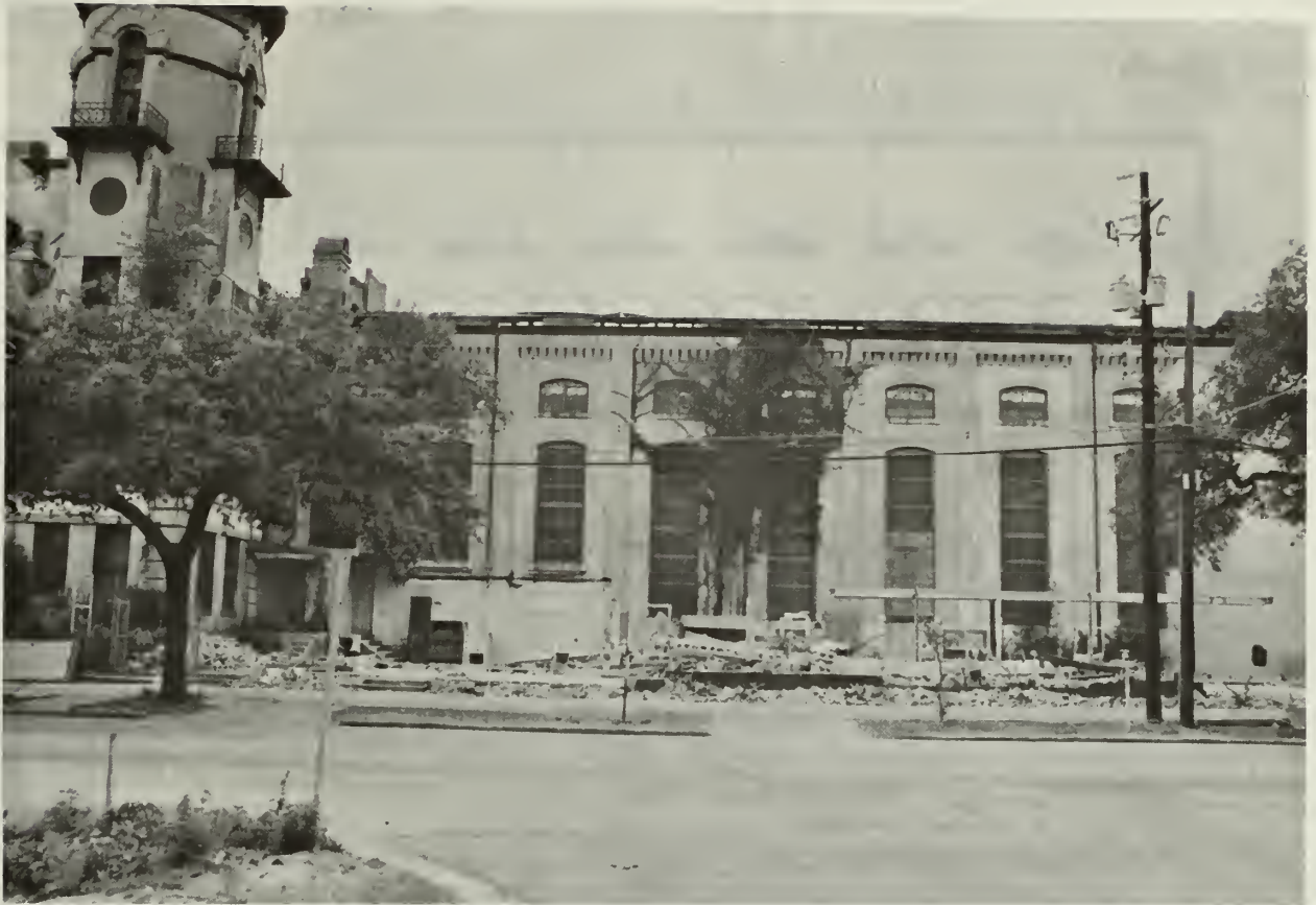
1. The property undergoing rehabilitation consisted of a three-story warden's house (partially visible, left) and a four-story cell block.
