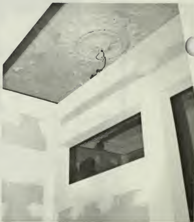
6. Work in progress: Center parlor. New partition wall for kitchen designed not to abut historic ceiling, yet is centrally located in room
