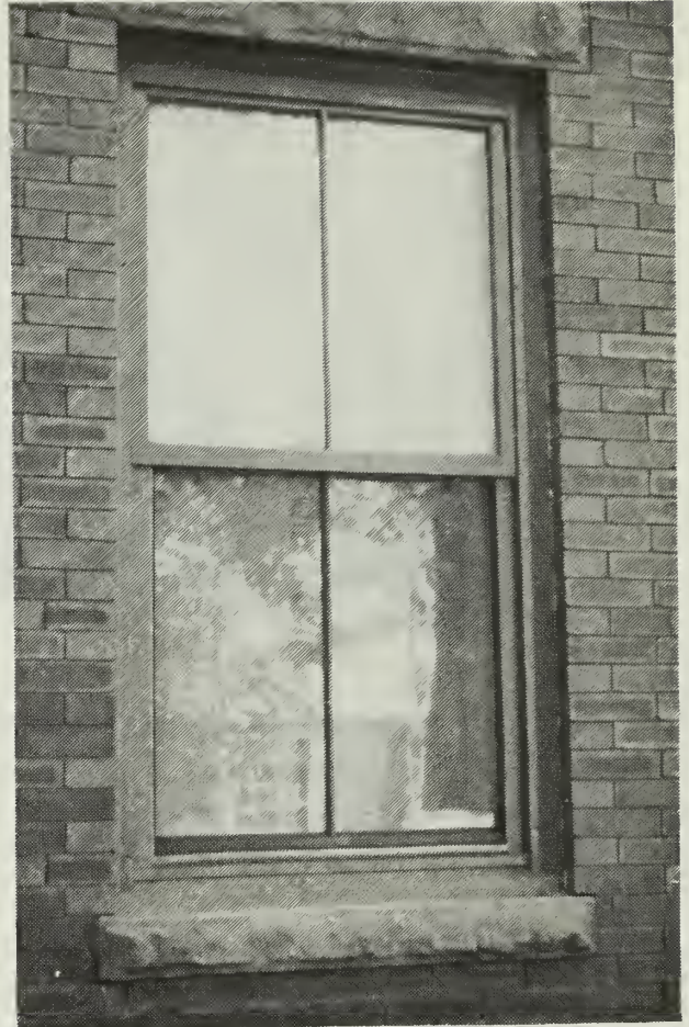
4. Aluminum replacement window with a wood mock-up of an applied unglazed sash frame and muntin placed over the upper aluminum sash. The applied frame and muntin look like temporary add-ons, rather than matching the historic sash.
