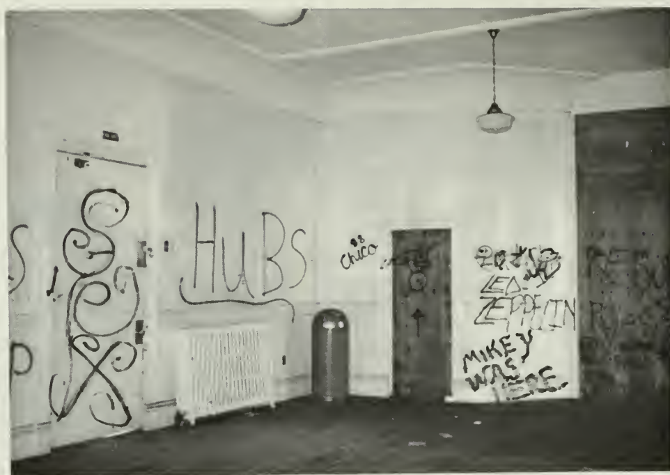
3. Interior view of ticket booth prior to rehabilitation. This historic feature was removed in the process of rehabilitation.
