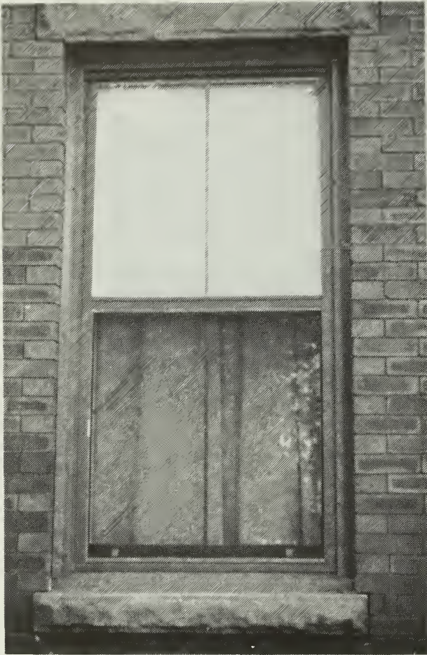
3. Post-rehabilitation photograph of aluminum replacement window. The vertical muntin was sandwiched within the insulating glass and the double-hung appearance changed since the screen panel was installed directly below the fixed upper sash.
