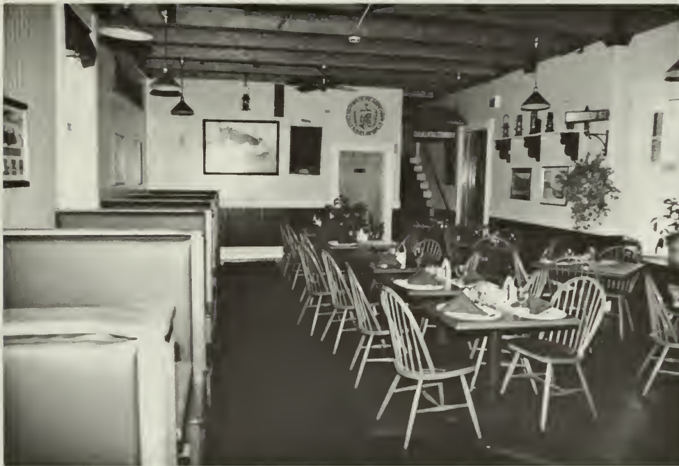
5. Post-rehabilitation view of waiting room. Note the removal of existing ceiling, and the addition of exposed ceiling joists above.
