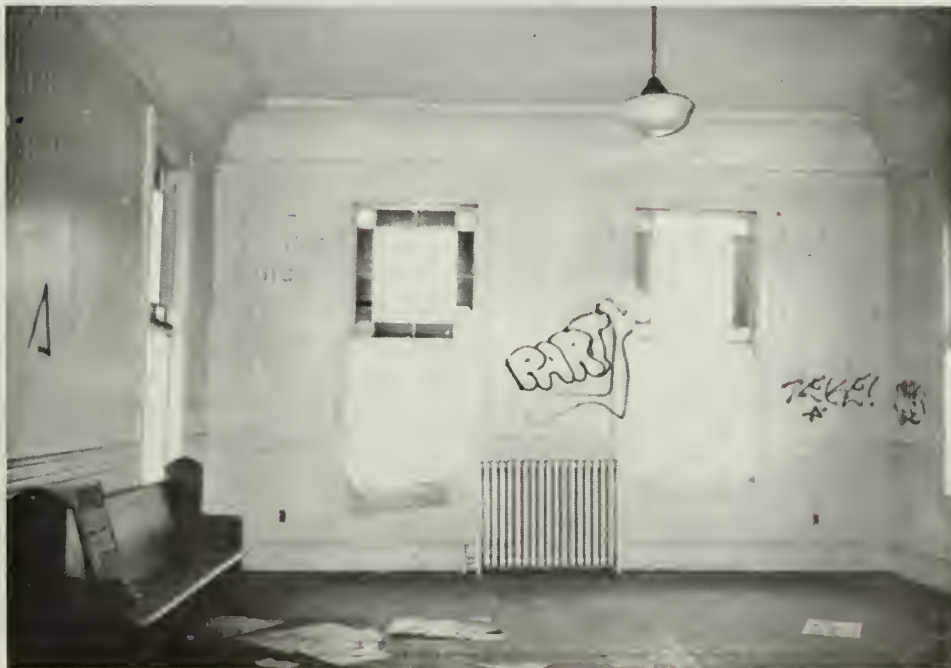
2. Interior view of waiting room prior to rehabilitation. Note wooden ceiling and wide covered cornice.
