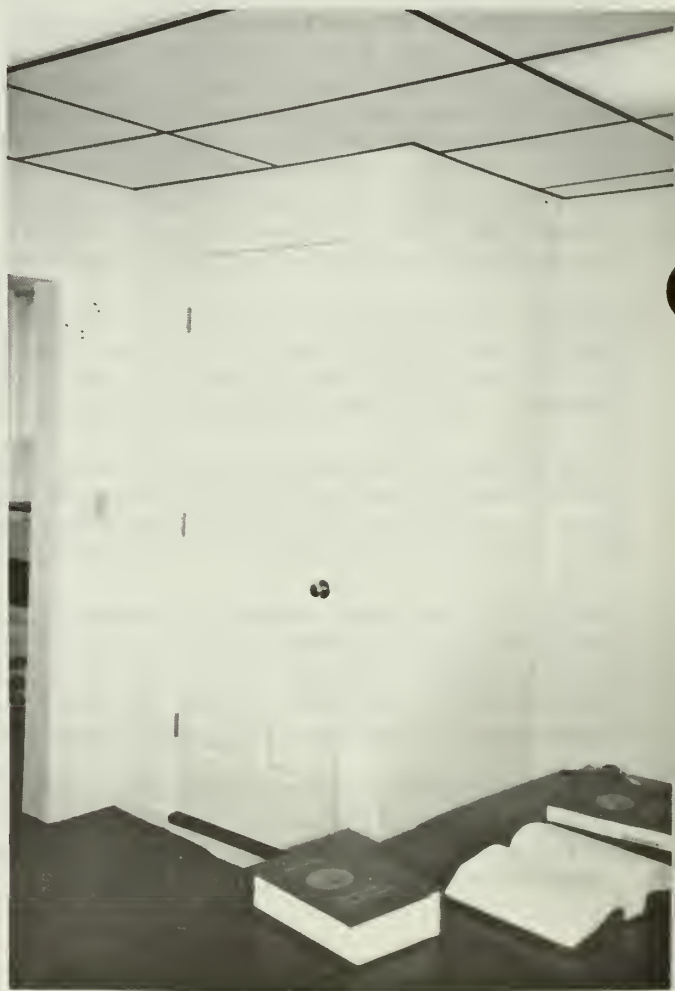
2. This view shows the distracting metal grid and ceiling illumination of the new dropped ceiling.
