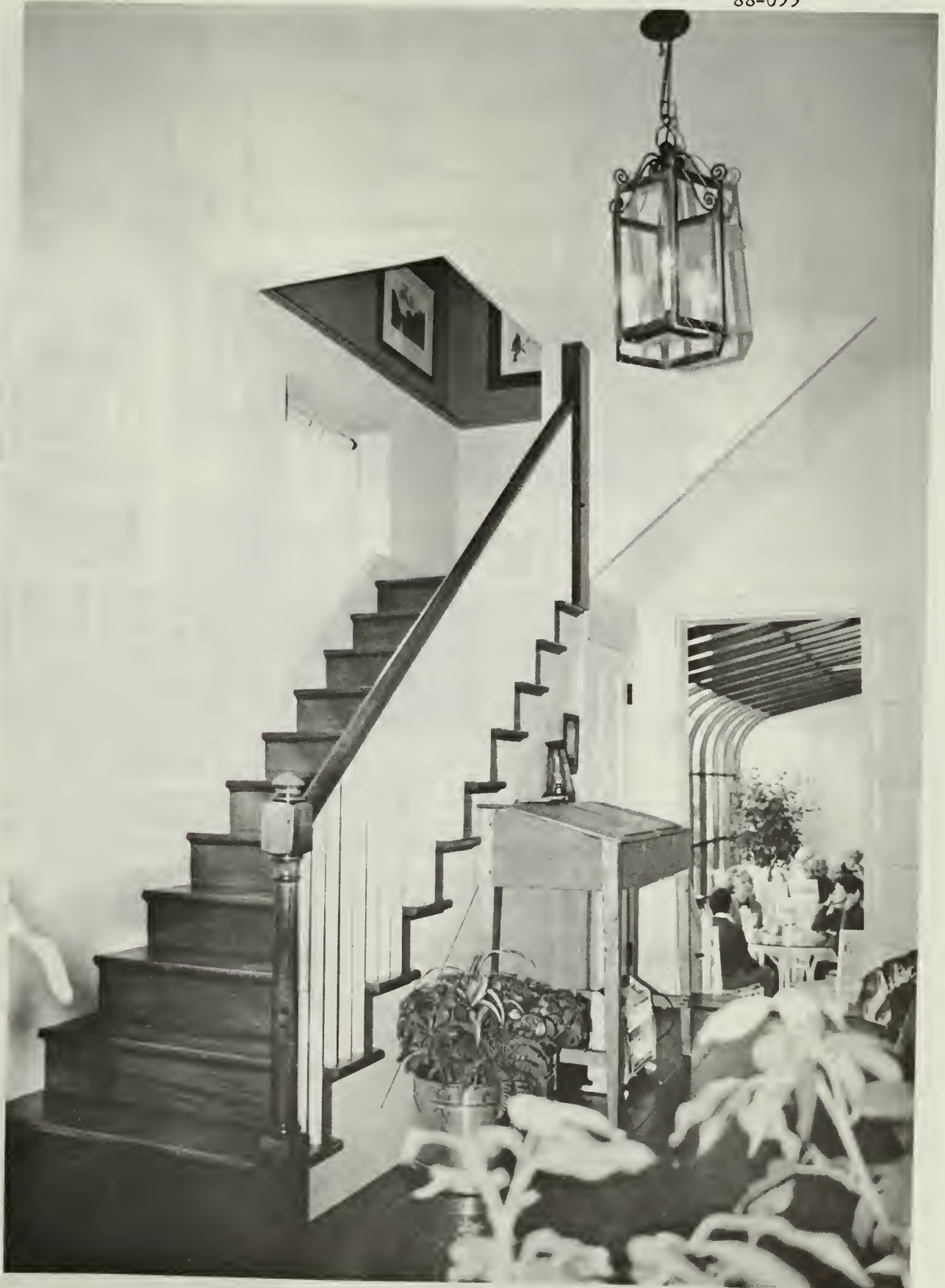
3. New stair after rehabilitation. Design of stair was not based on historic evidence.
