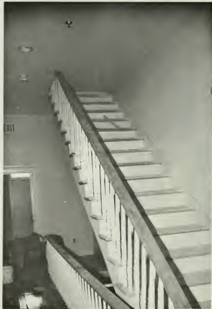
11. Post-rehabilitation view of original staircase maintained as a part of rehabilitation, but fourth floor is floored above, preventing access.
