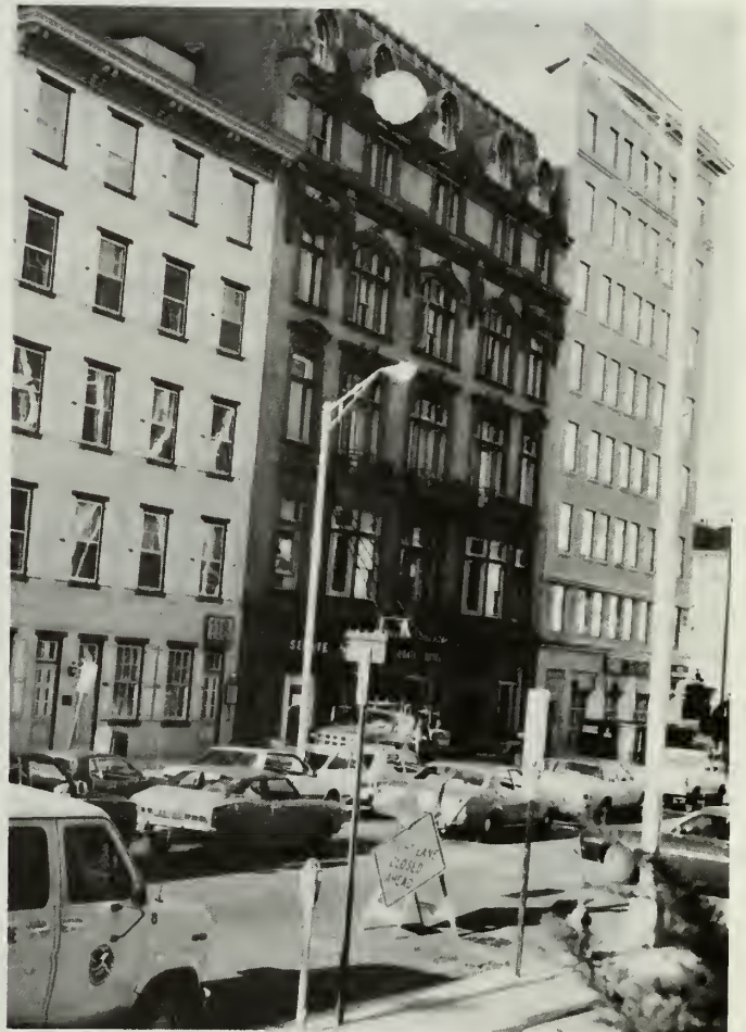
2. During rehabilitation into an office building the first floor is being reconstructed according to the original architectural drawings.
