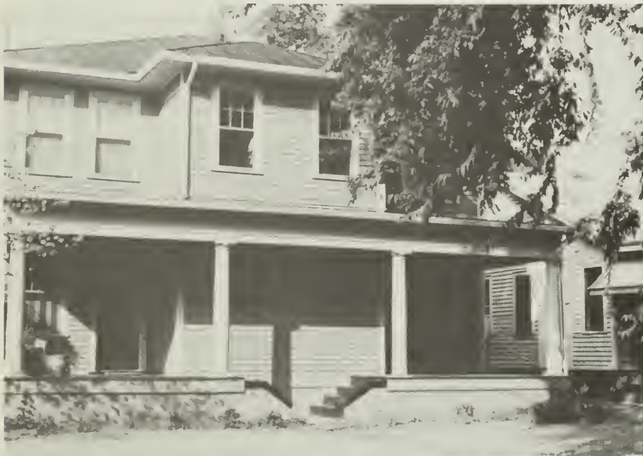
2. In connecting the two historic porches, the twin porch design was lost; a strong horizontal element was created by the large continuous porch; and the sense of a duplex building was diminished. To obtain certification, the owner agreed to restore the porch.
