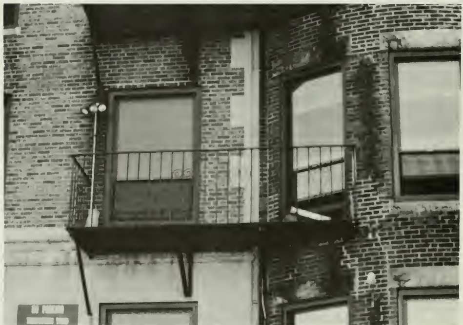
2. This is a close-up view of the contemporary window units which were installed. They had flat framing detail, bronze-anodized finish, tinted glass, and a lowered meeting rail.
