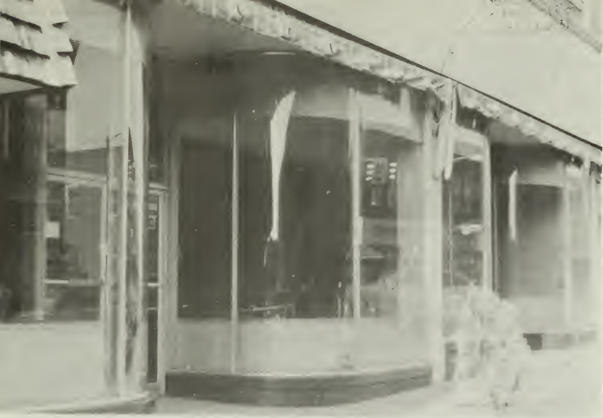
3. The entire storefront was replaced following breakage, during rehabilitation of one of the curved sheets of glass. Expediency and difficulty in locating a manufacturers of curved glass were cited by the owner as reasons for the change.
