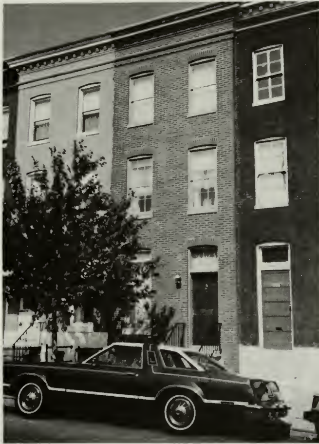
3. Brick rowhouse in center after paint removal using sodium hydroxide stands out conspicuously from its still painted neighbors.
