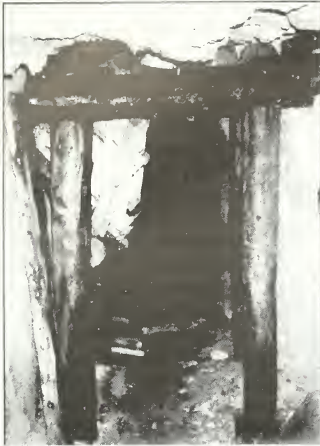
Figure 5.10. Support timbers in the underground workings of the Lucky Girl Mine, such as this square set in the No. 3 Adit, indicate considerable deterioration. The stulls are waterlogged and subjected to annual freeze-thaw cycles. Photo by Logan Hovis, 1998; on file at park office.
