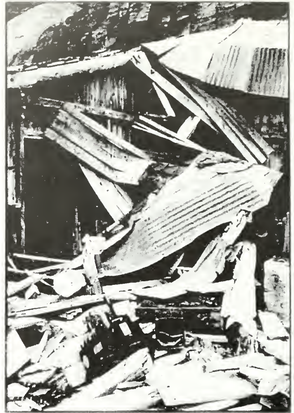
Figure 6.1. Few measures could lessen the destructive force of large slides. The compressor room at the Lucky Girl Mine has lost much of its structural integrity, although the extended roofline, covering dead space between the back wall of the building and the cliff face remains intact. Photo by Patrick Martin, MTU #BL-3.9.98.
