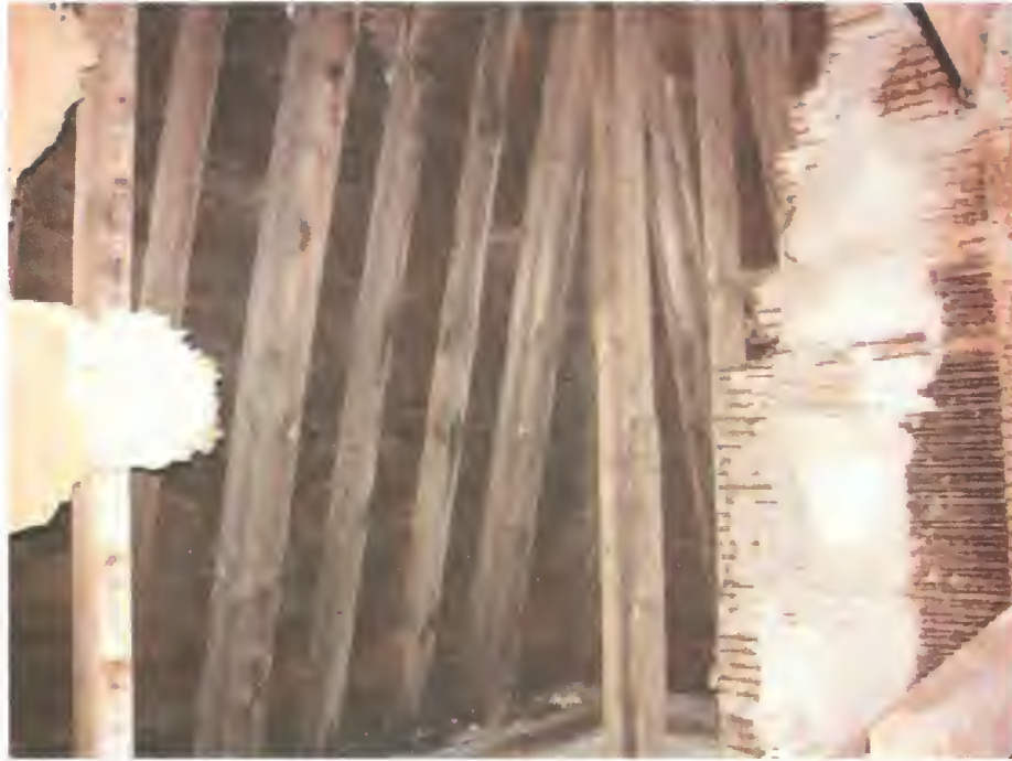
Figure 40. Officers Club, attic, showing framing of lower slope of mansard roof with alternating jack rafters, 2005.
