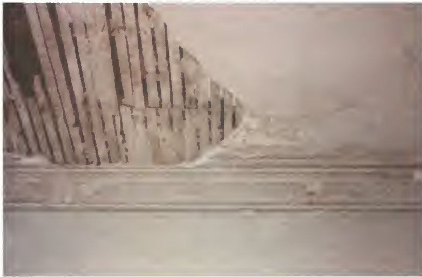
Figure 46. Officers Club, second- story center hallway (Room 201), ceiling plaster on wood lath, 2005.
