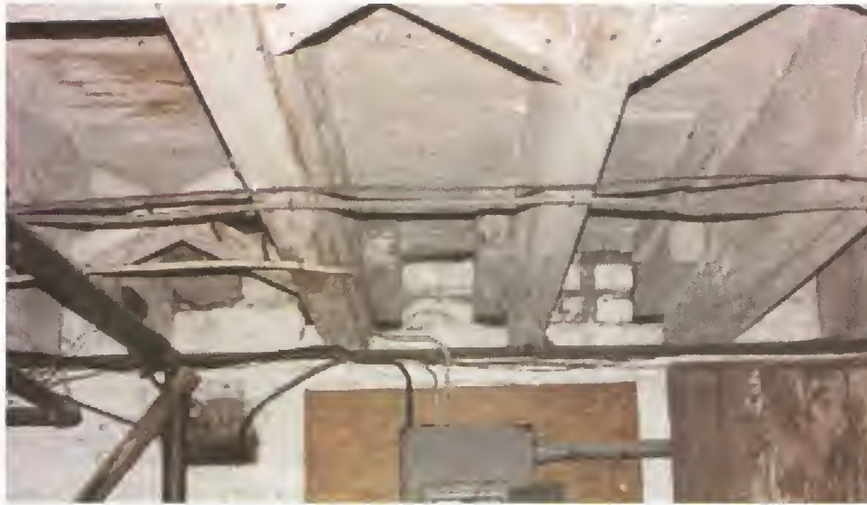
Figure 30. Officers Club, basement of rear ell, south wall, showing extant framing and brick infill that is evidence of earlier opening, 2005.
