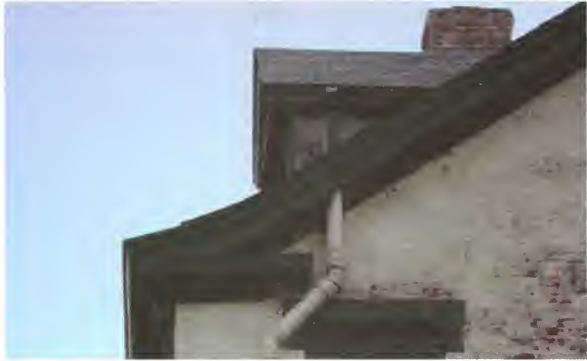
Figure 53. Officers Club, west elevation of rear ell, flared eave of ca.- 1905 addition, 2005.
