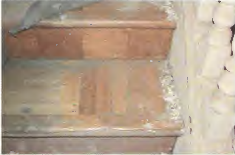
Figure 44. Officers Club, center hallway (Room 102), stairway, showing parquet pattern on treads and risers, 2005.
