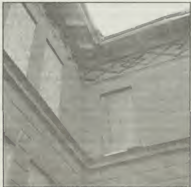
Figure 101. Detail, Vine Street School, showing wide eaves with beltcourse, and rusticated walls. Sebald.
