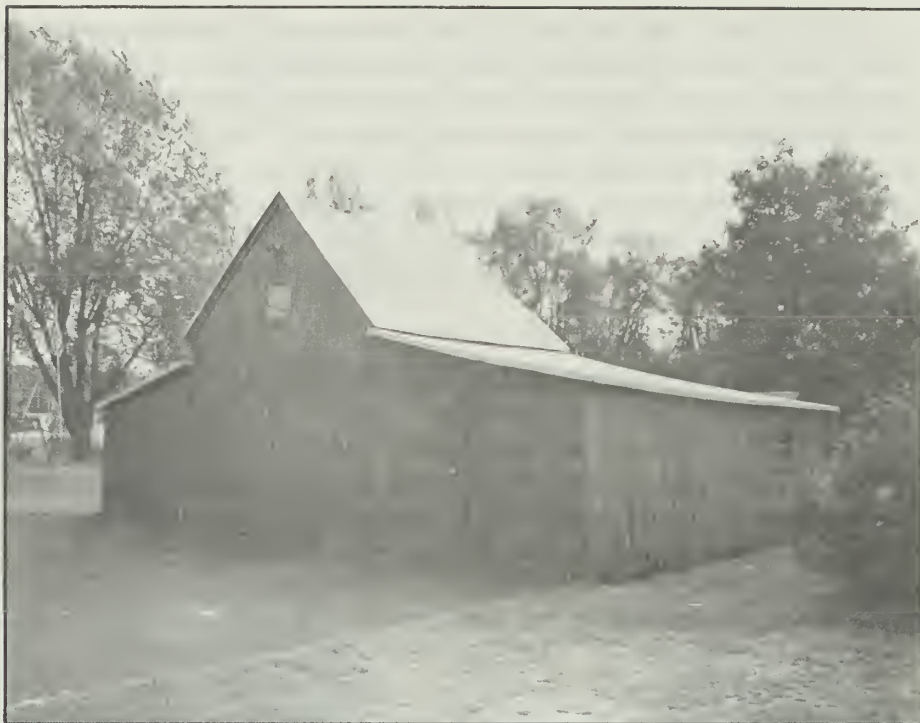
Figure 47. The drive-in corncrib form, here adapted for use as a garage, housed grain in the flanking compartments; the gable-end opening has been glazed.
