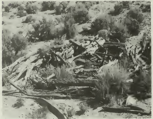
Collapsed cribbed-log hogan.
