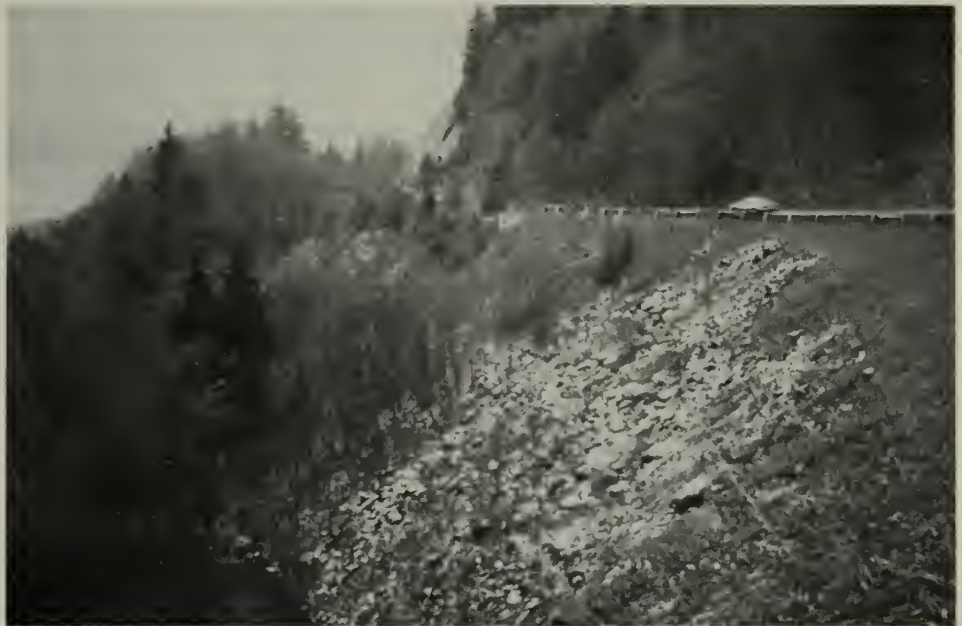
Site of roadcut and Anakeesta road-fill placement above Beech Flats Creek in GSMNP.
