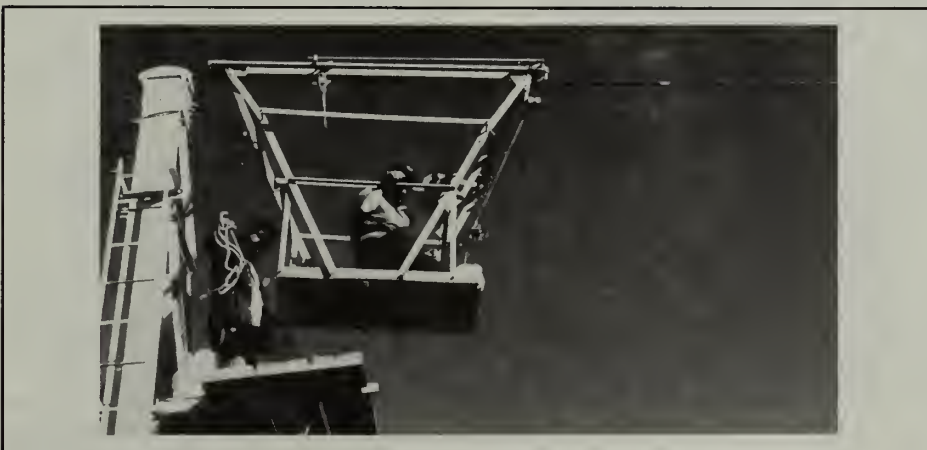
Cableway, used in synoptic experiments for water sample collections on the Colorado mainstream.
