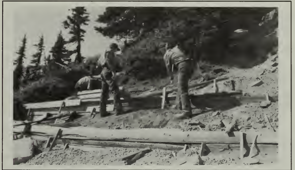
Restoration crew is shown here installing stabilization bars or silt dams; the area in the foreground has been filled with gravel and will next be filled with soil.
