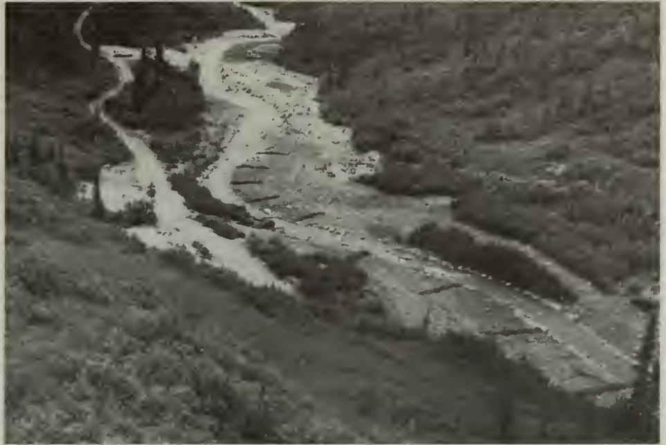
Brush bars for floodplain stabilization may be seen on either side of the channel in this aerial view of the lower half of the 1991 study reach on Glen Creek in Denali NP.
