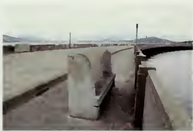
Figure 91. Historic concrete bench, parapet walls and curbing, light standards, and other site features associated with the Municipal Pier. (NPS, 2007)
