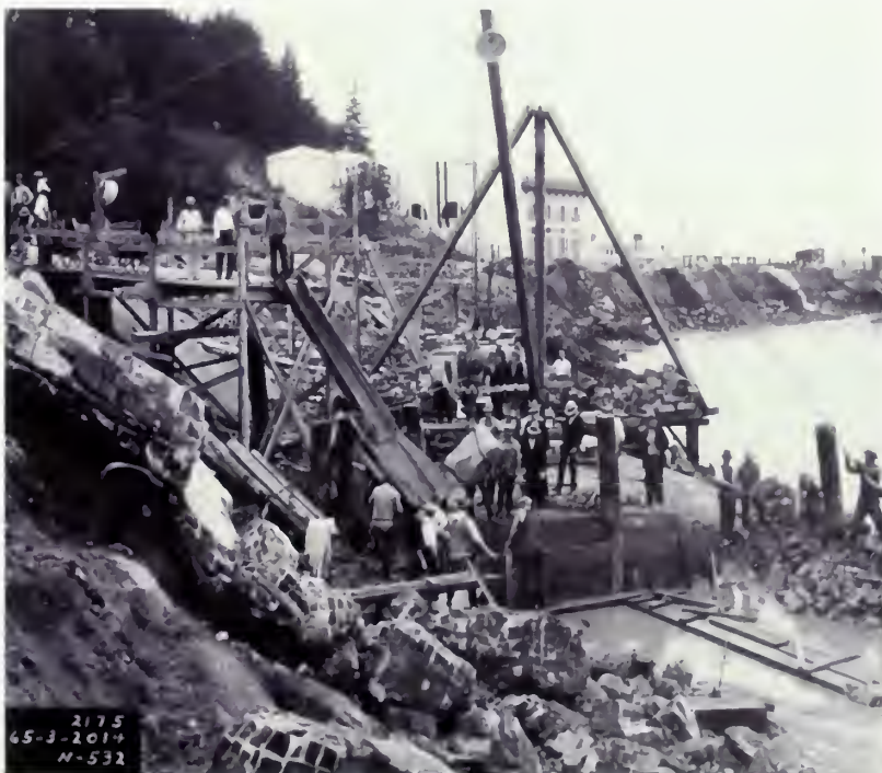
Figure 12. Detail of WPA photograph showing work crews using derricks, pulleys, and other devices to place large stone for the foundations of structures built around the cove. Note the building debris dumped on the slope for use as fill. View looking west ( San Francisco Maritime NHP, Historic Documents, Photograph Collection, P88-035.00007 )
