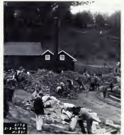
Figure 11 Collected from city improvement projects, a variety of salvage materials were brought to the site and used as fill material. View looking west. ( San Francisco Maritime NHP, Historic Documents, Photograph Collection, P88-035.00027 )
