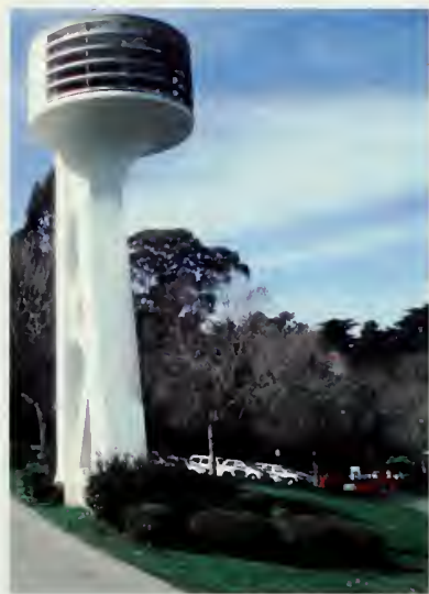
Figure 76. Grecian laurels ( Laurus nobilis ) remaining around the West Speaker Tower. View looking west. (NPS, 2008)
