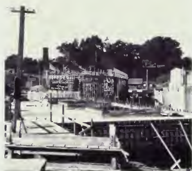
Figure 18 By February 1937, crews were framing and completing concrete work for the upper floors of the Bathhouse. ( San Francisco Maritime NHP, Historic Documents, Photograph Collection, P88-035.00074 )
