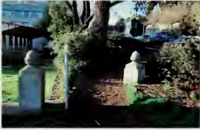
Figure 97. Remnant features of the original stone retaining wall as it wrapped around the park to Van Ness Avenue. View looking south. (NPS, 2008)
