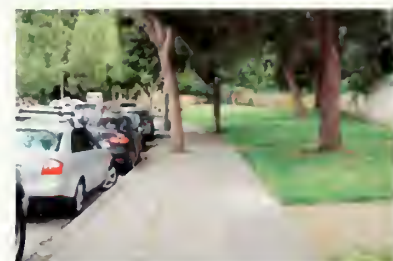
Figure 108 Displaced, cracked, and patched sidewalk along Van Ness Avenue next to Pocket Park. At a certain point, rather than patching, a holistic approach to rehabilitation of the sidewalk will assure a more uniform character. View looking south (NPS, 2008)
