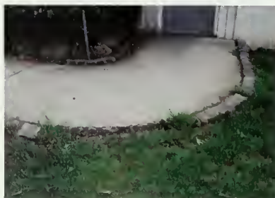
Figure 94 Missing block curbing at the West Convenience Station should be repaired using in-kind materials. (NPS, 2007)
