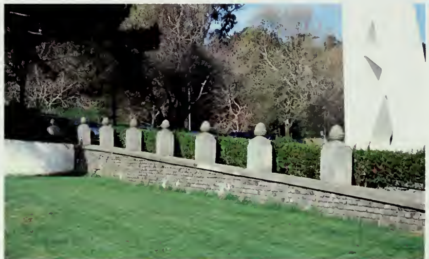
Figure 98. View of the stone retaining wall looking northwest from the lawn near the Bocce Ball Courts. The amount of exposed wall visible in the park today generally slopes to the east based on fill added to even the grade when the pump house was removed in the 1940s. (NPS, 2008)
