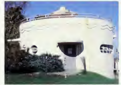
Figure 92. Staining on the exterior of the West Convenience Station. (NPS, 2007)
