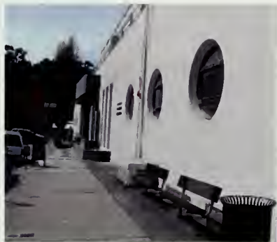
Figure 88. Northeast side of the entrance to the Bathhouse with a variety of non-compatible features such as benches, trash cans, city street signs, utilities, and public mailbox. (NPS, 2010)
