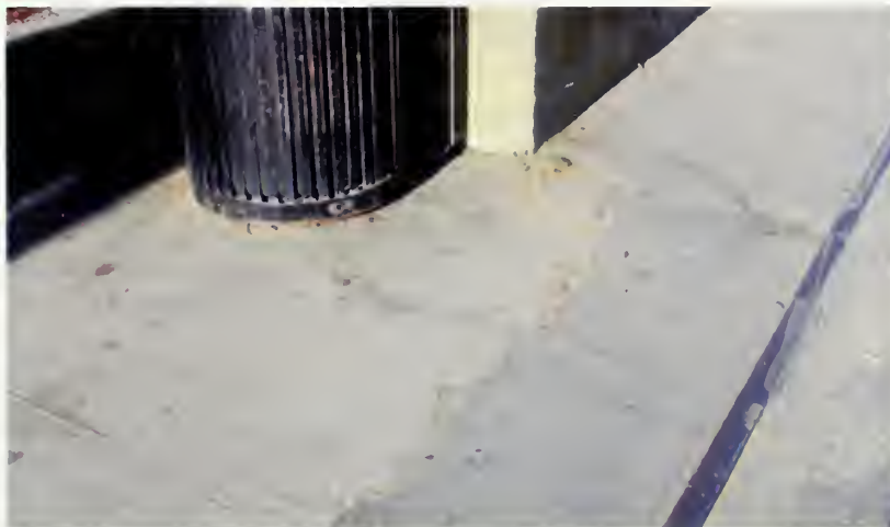
Figure 100 In some areas walkways have been resurfaced with paving added over existing layers creating a patchwork of materials. (NPS, 2008)
