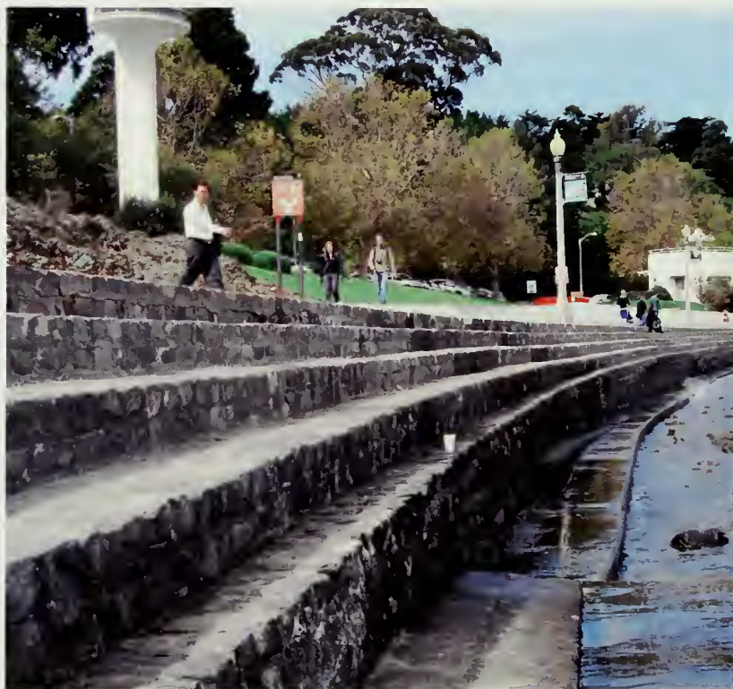
Figure 93. One of the earliest structures built during the historic period, the Seawall around the cove is in relatively stable condition. (NPS, 2009)
