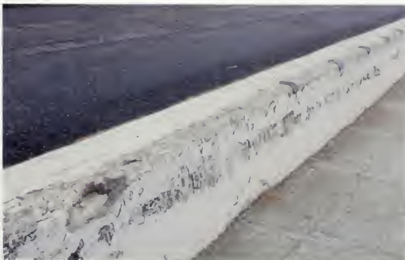
Figure 96 Flaking and loss of material along the concrete wall occurs as deterrent bolts fail and water penetrates the under layers of the concrete. Repair may require patching, reapplication of a skim-coat, or some combination. View of the east end of the wall, looking west (NPS, 2007)
