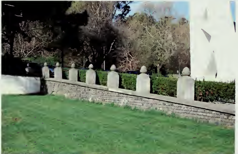
Figures 67. Stone masonry retaining wall as it appears today near the Bocce Ball Courts. A considerable amount of backfilled was used after the pumping station was removed to create a level grade on the south side of the structure. View looking west towards Van Ness Avenue. (NPS 2007)
