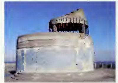
Figure 65 The unfinished convenience station at the end of the Municipal Pier (NPS, 2007)
