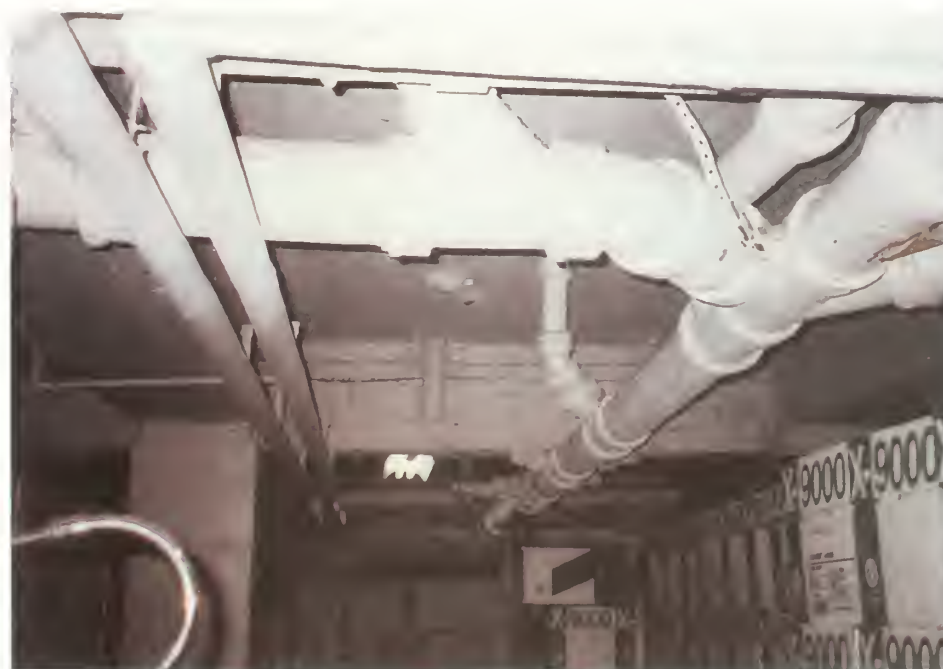
Figure 77. North side of basement, center of ceiling, showing concrete slab flanked by concrete beams (added to support concrete floor in first-story lavatory).
