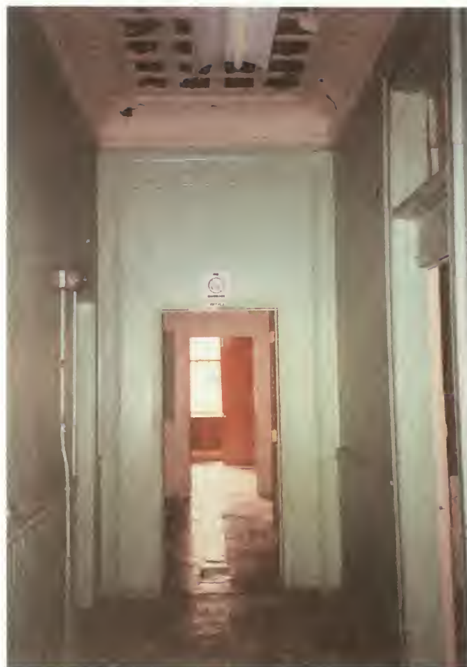
Figure 79. Doorway from side hall to mess room, showing perimeter infill for replacement door and covered transom.
