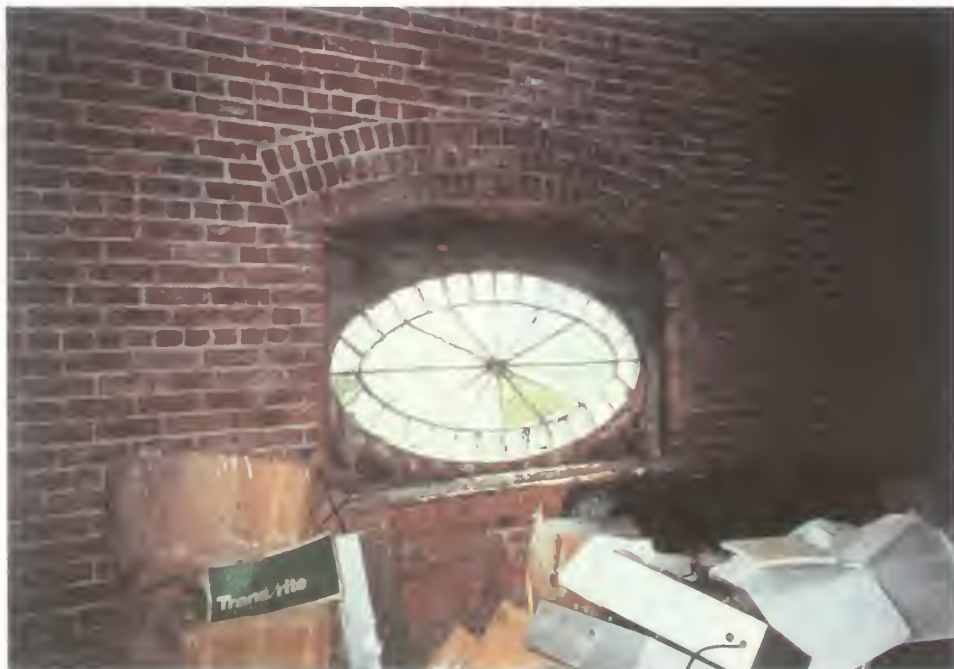
Figure 83. South side of attic, south wall, showing interior construction of opening for oculus.
