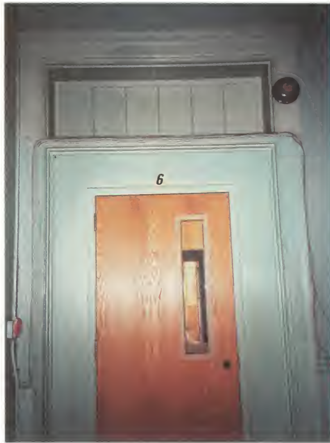
Figure 82. Doorway from center hall to south dormitory, showing perimeter infill with replacement door, and painted transom.
