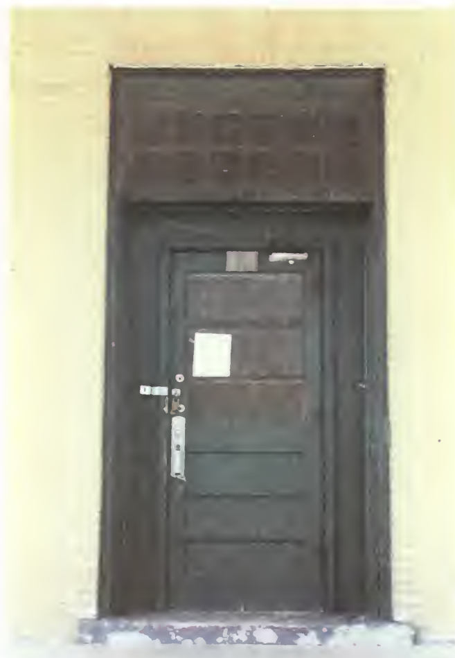
Figure 75. East elevation, first-story doorway, showing perimeter infill with replacement door, and original transom.
