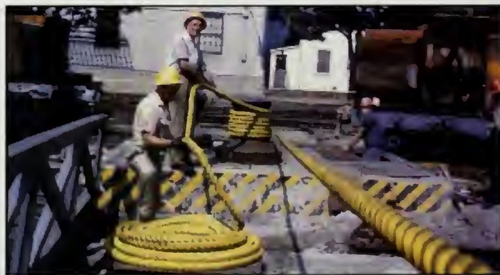
CAPSTAN — The Navy Yard utilized electric capstans to assist maneuvering ships in its dry docks. Here workers play out nylon rope being wound around the capstan at the head of Dry Dock 2 in the early or mid-1960s.
