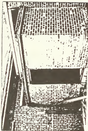
26. Northwest pump house. Note severely cracked brick walls.
