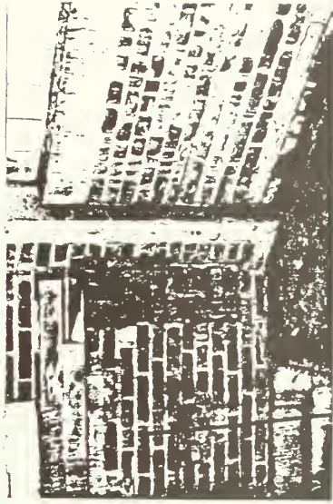
11. View of interior water damage at west tower.
