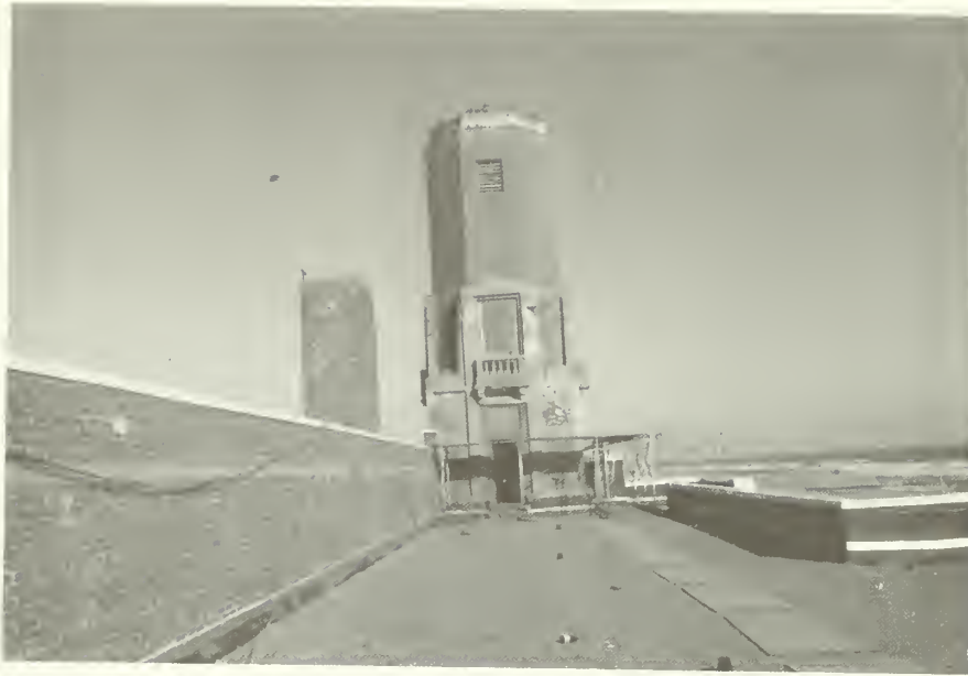
Figure 11: Built-up roof of Part 2 looking east. Worn areas of roof found to have water below surface of felt. East Tower in background. NPS photo, October 1985.
