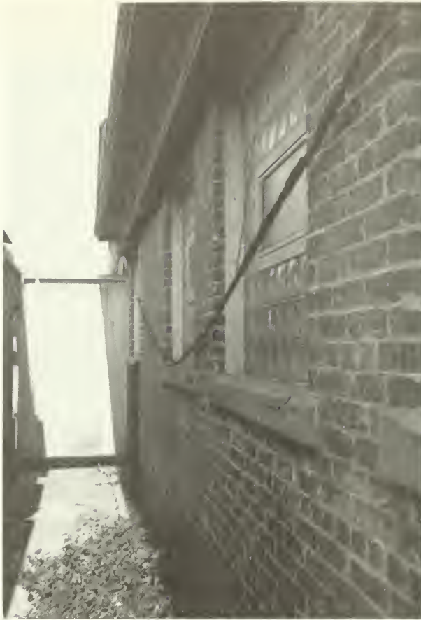
Figure 75: West wall of East Wing, showing typical eave and sill conditions. NPS photo, 1985.
