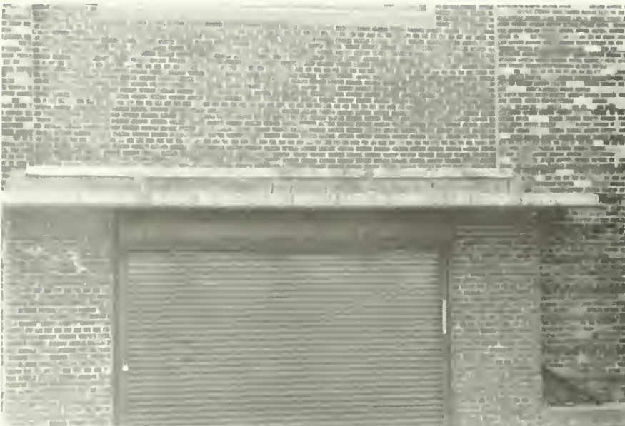
Figure 20: Typical oxide jacking at concrete canopies. Rust and steel bars visible. Typical rollup doors below canopy. NPS photo, October 1985.
