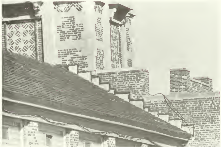
Figure 10: Rusting drip flashing at roof edges, West Tower. Note cornice and eaves below, and faulty counterflashing at base of tower. Tar at joints of flashing is deteriorating. NPS photo, October 1985.
