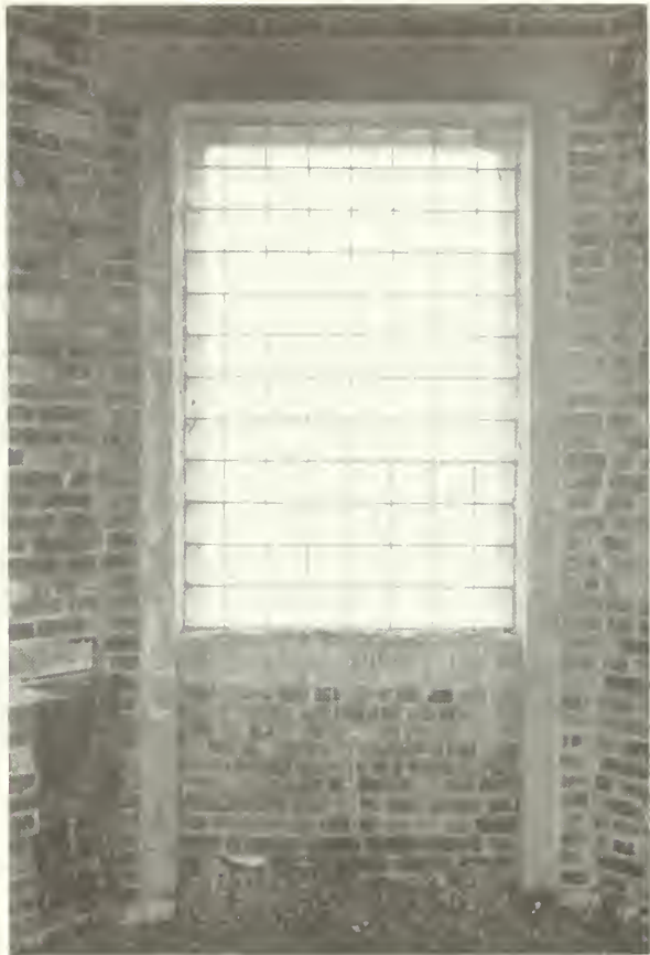
Figure 29: Solid glass block masonry openings and damp walls in towers. Note pigeon waste at floor. NPS photo, October 1985.
