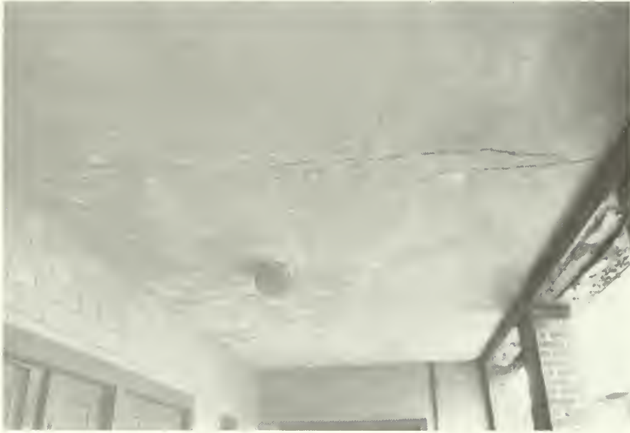
Figure 71: West Wing loggia, cracks in ceiling. NPS photo, 1985.
