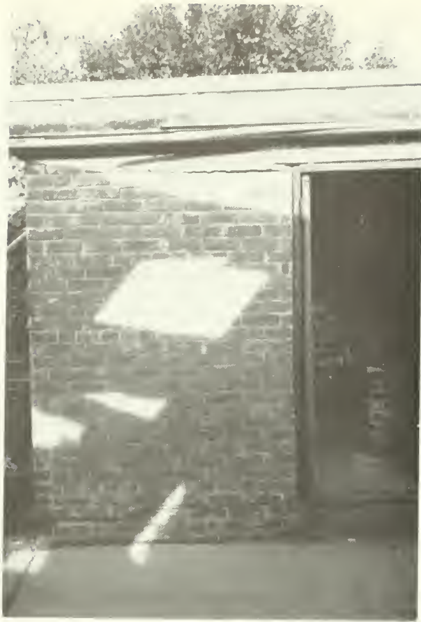
Figure 63: Meter Room at East Screen Wall. NPS photo, 1985.
