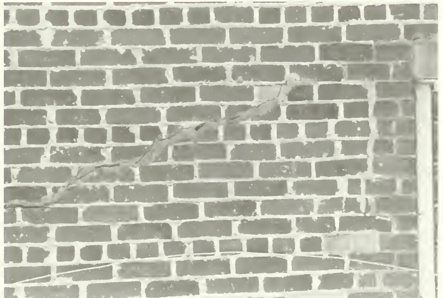
Figure 22: Typical condition of repaired cracks. Cracks are reopening. NPS photo, October 1985.
