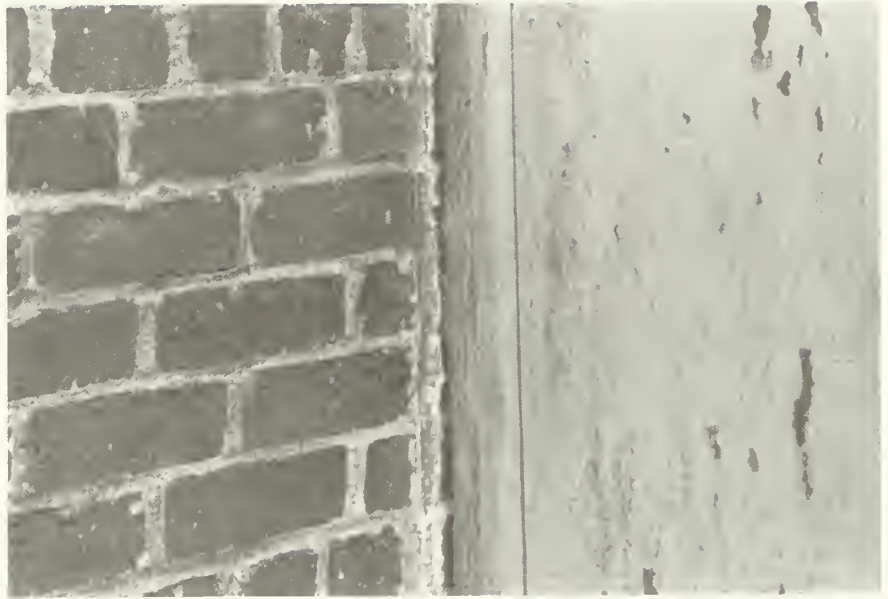
Figure 17: Sandblasted wall outside of "Shed A" (see Existing Conditions drawings). Shed walls to right. NPS photo, October 1985
