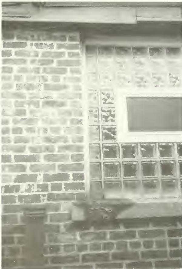
Figure 80: Dark stain and waxy efflorescence at Window 618, East Wing. NPS photo, 1985.
