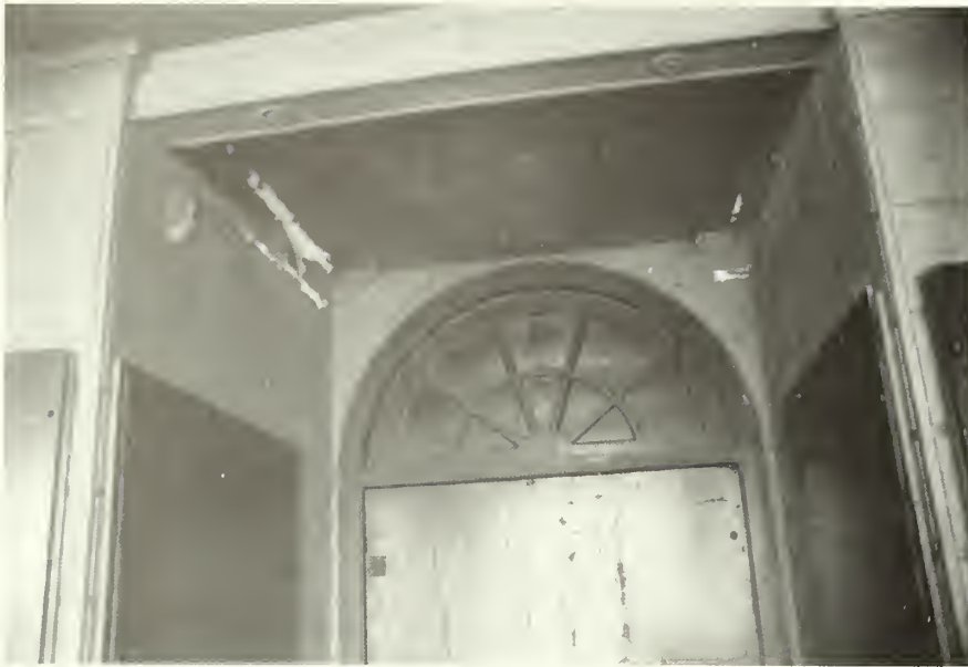
Figure 39: Plaster molding damage at door 410, Entrance Pavilion. NPS photo, 1985.
