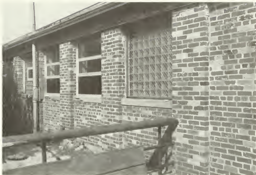
Figure 65: West Wing, West Elevation, showing spalling sills at windows 509, 510, and 511. NPS photo, 1985.
