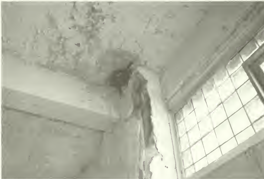
Figure 16: Moisture problems in kitchen area at beams, ceilings, and clay tile chase areas. NPS photo, October 1985.
