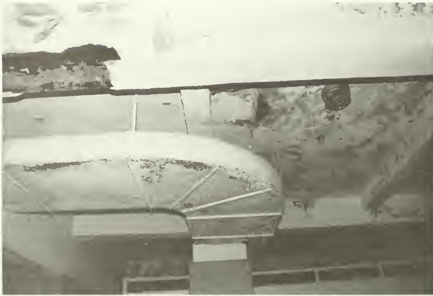
Figure 15: Other moisture problems in second floor area. Plaster and concrete coatings are spalling at beams and ceilings. Paint also blistering and peeling. NPS photo, October 1985.
