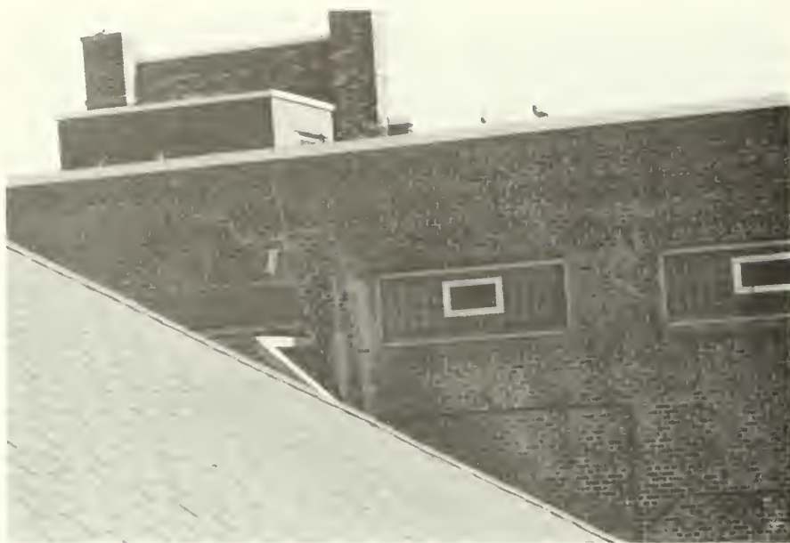
Figure 23: North elevation--part 2. Cracks typical at corners and in line of windows due to oxide jacking of steel lintels. NPS photo, October 1985.
