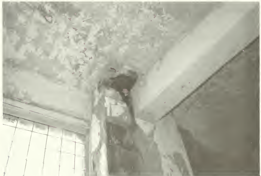
Figure 14: Water damaged plaster and clay tile chase in kitchen area. Problem caused by damaged roof leader. Other moisture around this area is attributed to poor ventilation and lack of temperature controls in the unconditioned space. NPS photo, October 1985.
