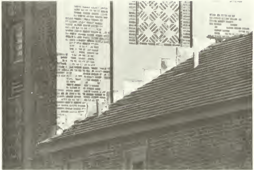
Figure 9: Faulty counterflashing at base of West Tower. Flashing pulling out from joints in wall. Joints needs repointing. NPS photo, October 1985.
