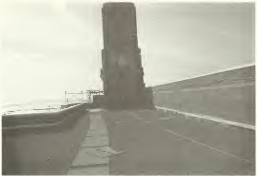
Figure 13: Built-up roof looking west. Worn areas indicate presence of water as on east side. West Tower in background. NPS photo, October 1985.
