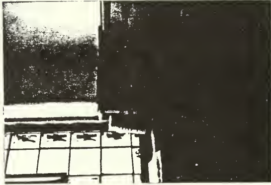
21. Settlement of east exterior wall of West Wing.
