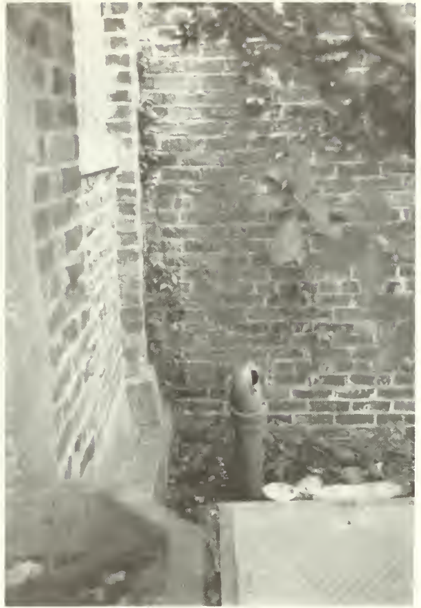
Figure 77: Wall bulging out under Window 631, East Wing. NPS photo, 1985.
