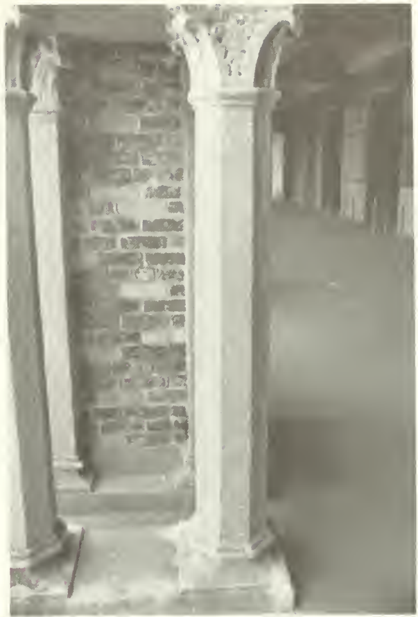
Figure 53: Typical cast stone columns, showing deterioration before patching. NPS photo, 1982.
