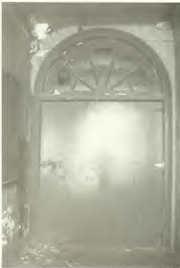
Figure 40: Plaster wall deterioration at door 409, Entrance Pavilion. NPS photo, 1985.
