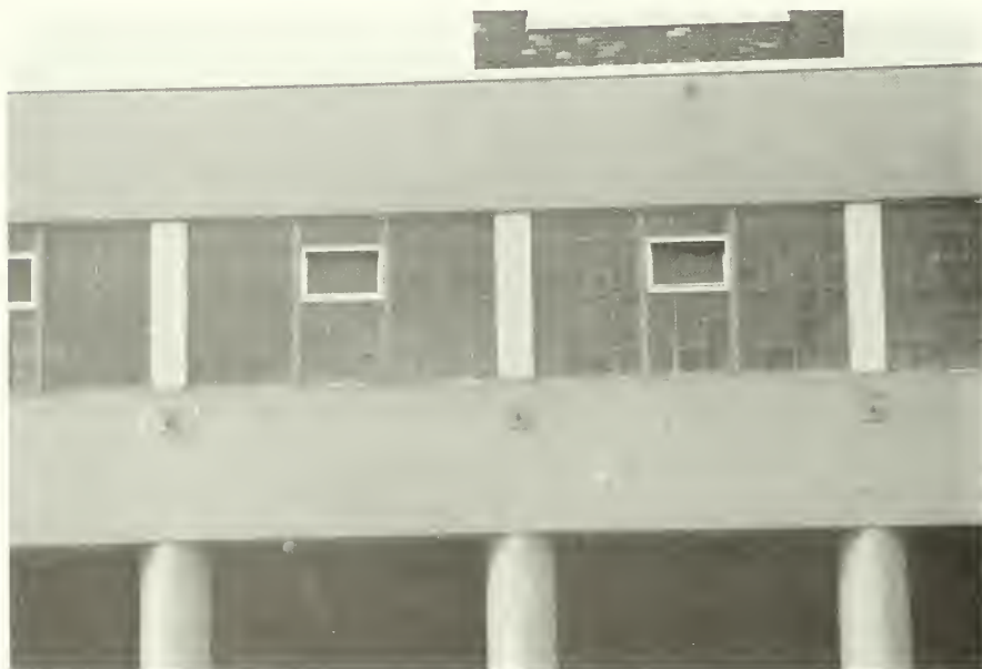
Figure 24: Elevation of loggia (North Elevation--Part 2). Note typical glass block windows with vents used throughout the Beach Pavilion. Problems of concrete in beams, columns and ceiling typical. NPS photo, 1985.
