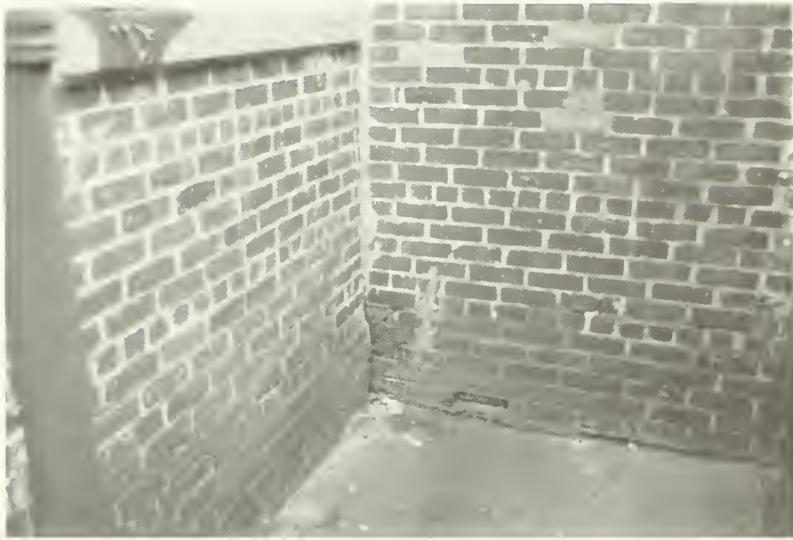
Figure 79: Wall bowing out under Window 618, East Wing. NPS photo, 1985.
