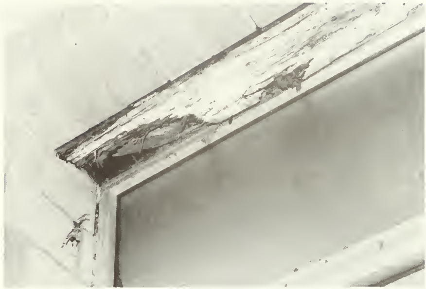
Figure 81: Rotten lintel at Window 629, East Wing. NPS photo, 1985.
