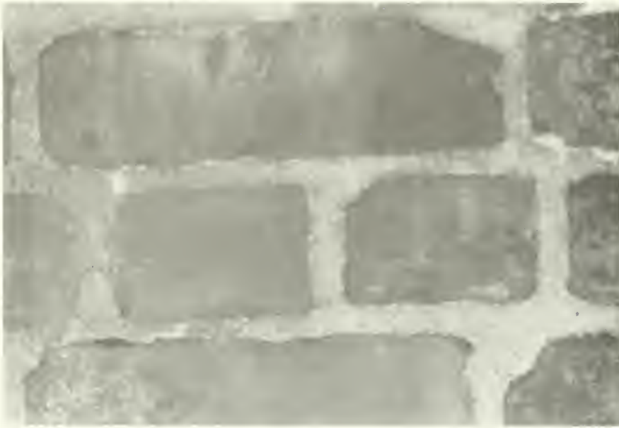
Figure 19: Closeup of unabraded wall beneath "Shed A." Note paint at mortar joints and on brickwork. NPS photo, October 1985.
