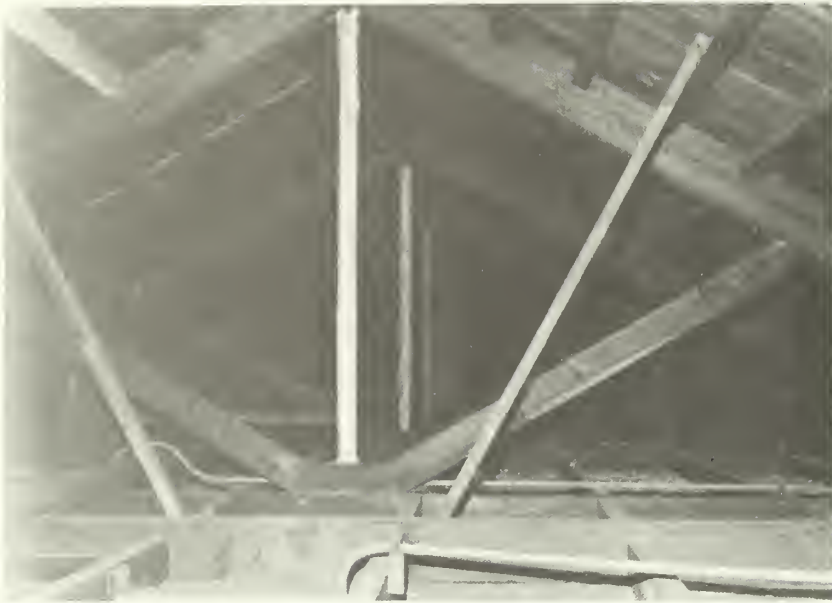
Figure 7: Roof framing at Beach Pavilion. Note wood trusses with steel central post. Ceiling framing below. NPS photo October 1985.
