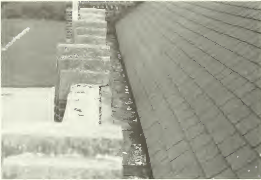
Figure 35: North gutter at Entrance Pavilion. NPS photo, 1985.
