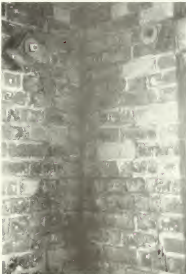
Figure 38: Typical wall conditions, with bolts at interior of Entrance Pavilion arcade. NPS photograph, 1985.
