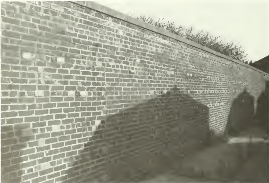
Figure 60: South face of East Screen Wall, showing brick infill at bay 9. NPS photo, 1985.
