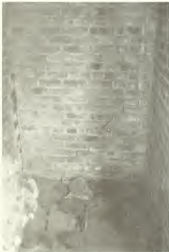
Figure 78: Interior of East Meter Room showing crack in west wall of East Wing. NPS photo, 1985.
