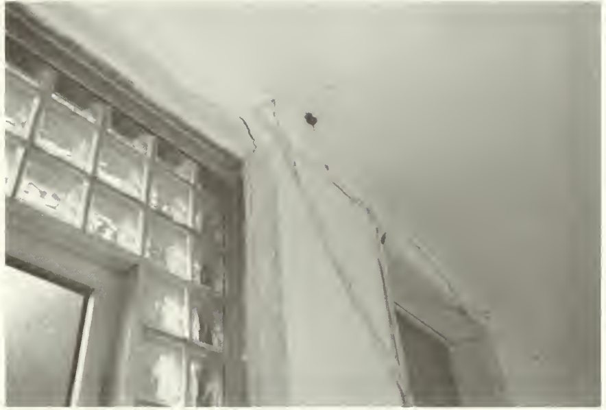
Figure 69: East wall bulging out, Windows 517 and 518, West Wing. NPS photo, 1985.
