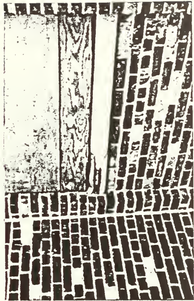
6. Typical cast stone deterioration at Beach Pavilion.
