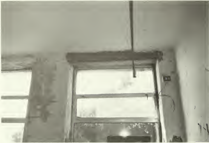
Figure 67: Water damage at Windows 510 and 511, West Wing. NPS photo, 1985.
