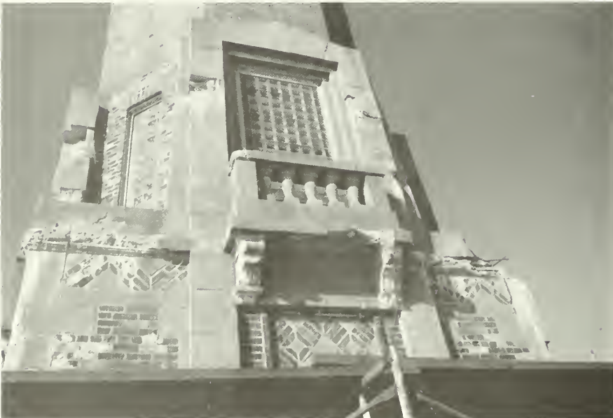
Figure 28: Deteriorating walls and decorative features at towers. Note also solid glass block windows. NPS photo, October 1985.
