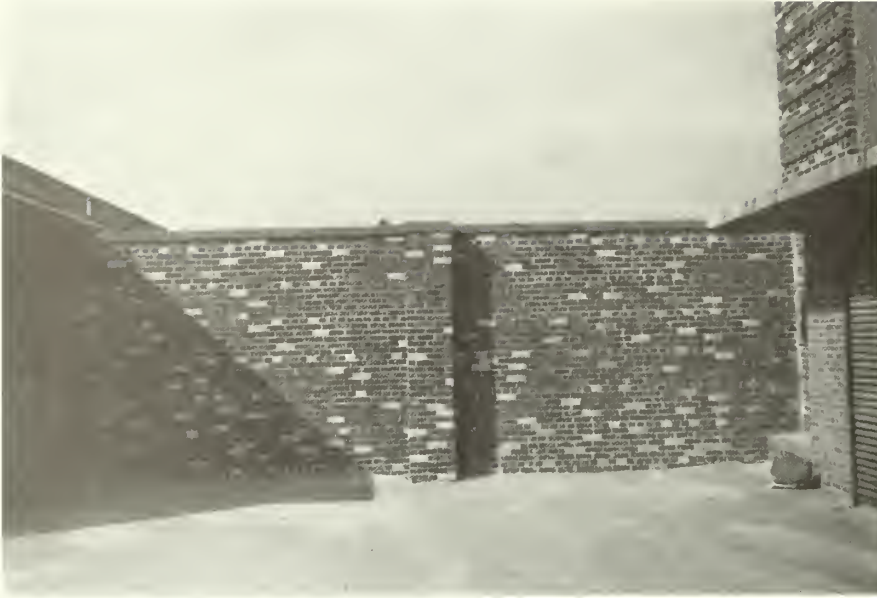
Figure 31: West Screen Wall: Masonry conditions typical to those of building walls (Pavilion). NPS photo, October 1985.
