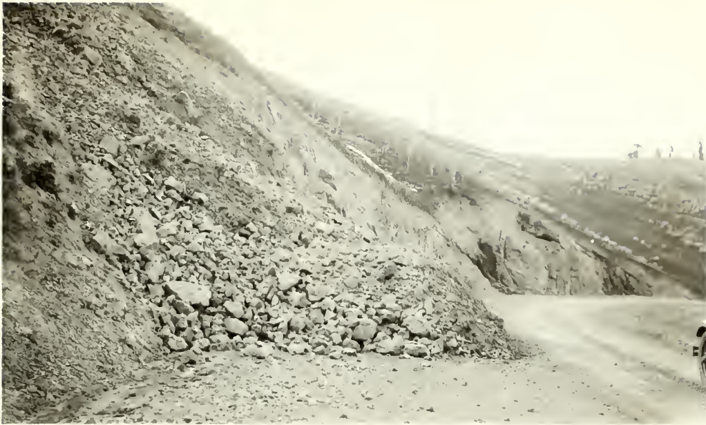
11130-6. Rock and mud slide on Dunraven Pass Road. This slide originally extended across the road but partially cleared away, project #348.
