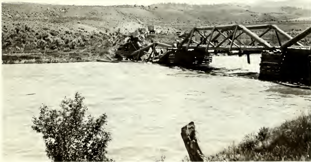
1119-1. One span of Lamar River bridge broken down by overload.
