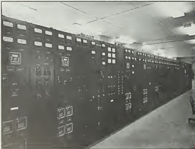
Figure 69: Interior view of control room, Building 20, 1991.
