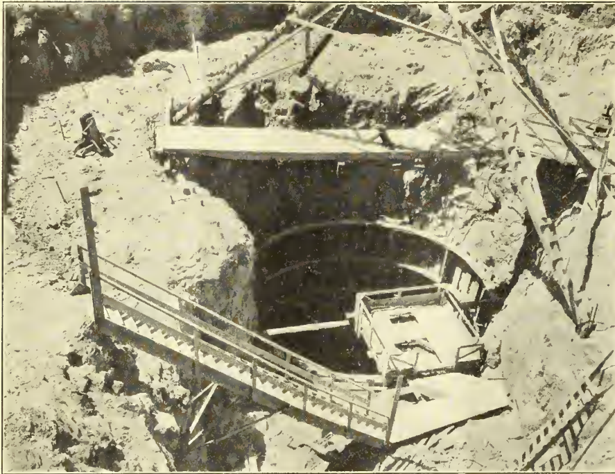
Glory hole at top of spillway shaft, Owyhee dam, Owyhee project, Oregon-Idaho
