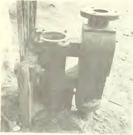
Figure 12. Reciprocal, steam-driven pump on tier 3.
