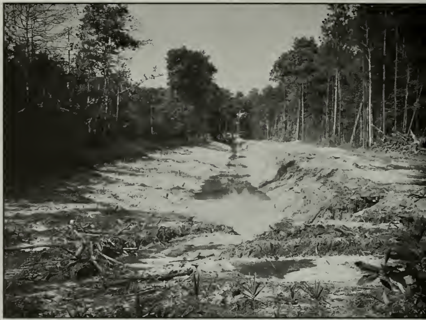
Figure 1. Construction of this drainage ditch in a housing development bordering the Davis Bayou Unit of Gulf Islands National Seashore was halted using provisions in Section 404 of the Clean Water Act. Water Resources Division and park staff showed that this ditch would have drained a valuable park pine savanna wetland (right).
