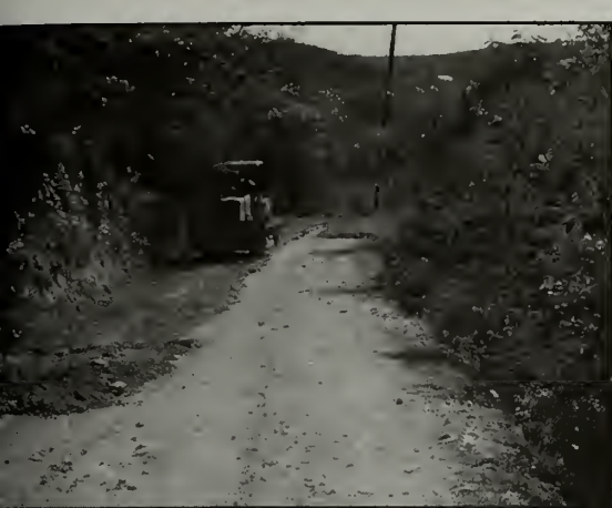
Approximately 50 km (31 mi) of unpaved roads, crudely bulldozed on steep terrain, Saint John Island; they provide a ready source of soil to be carried bayward during longer-rainstorms.
