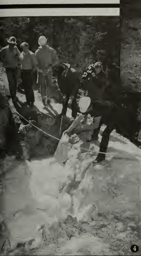
Figure 4. Installer directs expanding PUF foam into desired areas; Figure 5. The completed closure following earthen backfill.
