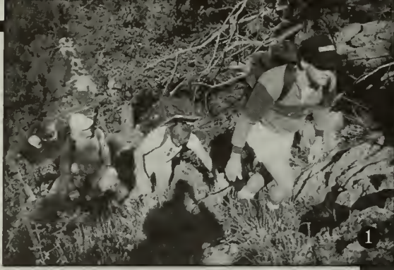
Figure 1. Volunteers backpack PUF kits into remote installation site; Figure 2. The PUF kit before breaking inner bag to mix with contents of outer sack; Figure 3. Installer builds support for PUF plug.
